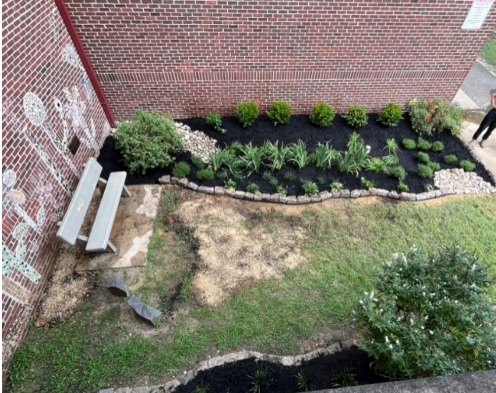
Rain garden installed at Thomas Edison Elementary School in Haddon Township, NJ
