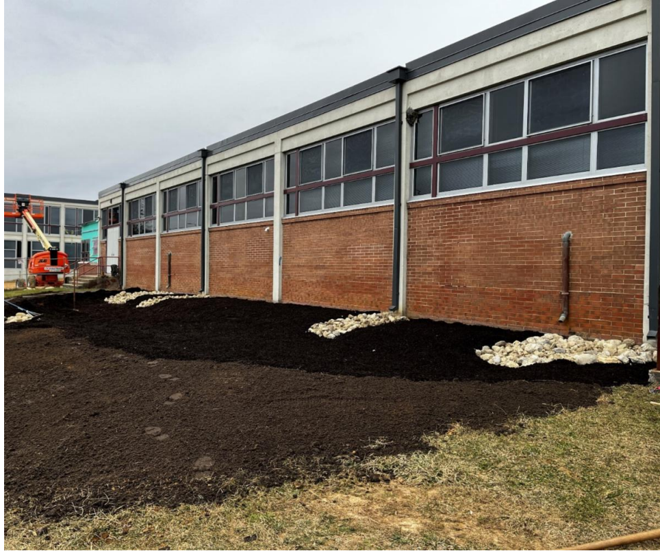
Rain garden construction at South River High School in South River, NJ
