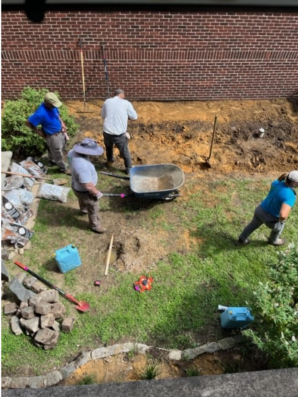
Rain garden construction at Thomas Edison Elementary School in Haddon Township, NJ
