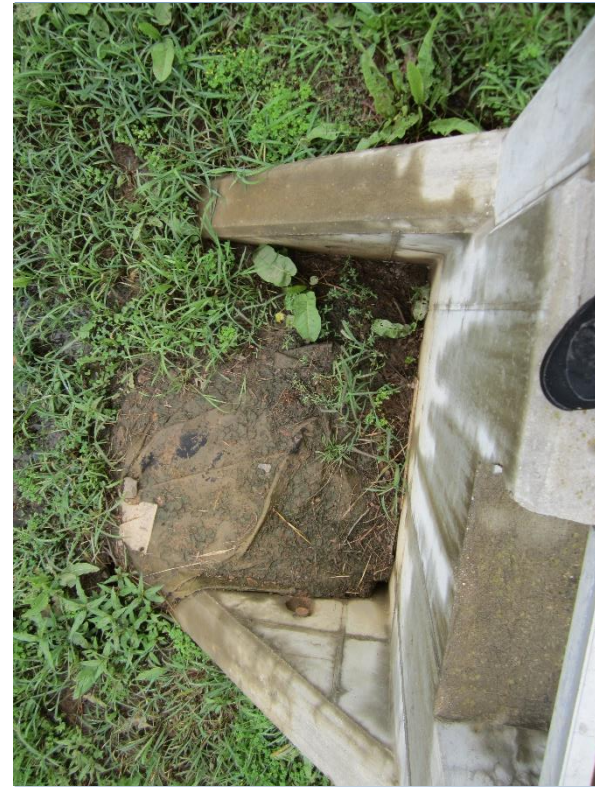
Outlet blockage by sediment
