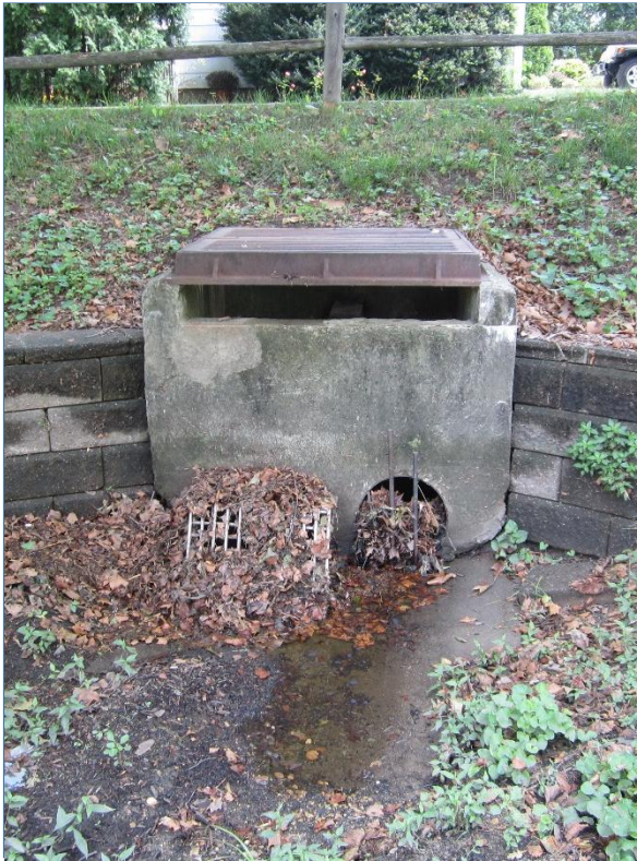
Outlet blockage by debris
