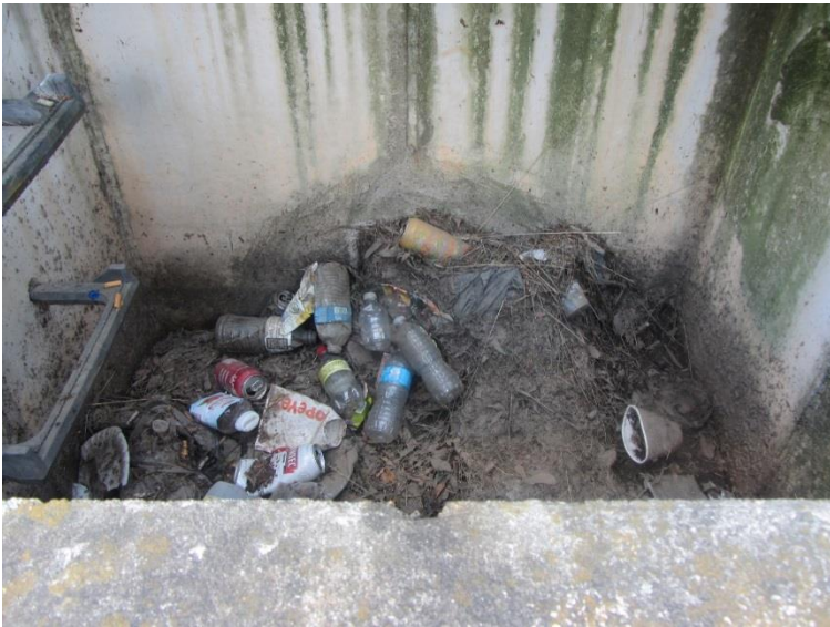
Accumulation of floatables from outfall
