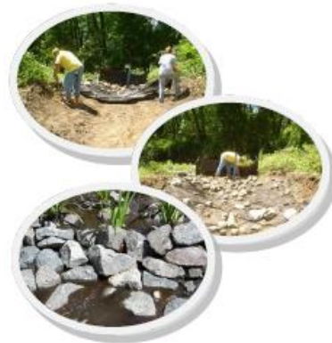
The rip-rap apron at the outlet provides for final settling and velocity reduction prior to entering the Troy Brook.
