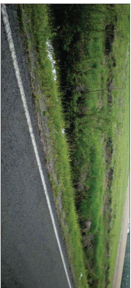
TYPICAL UNDERSIZED AND ERODING DITCH
