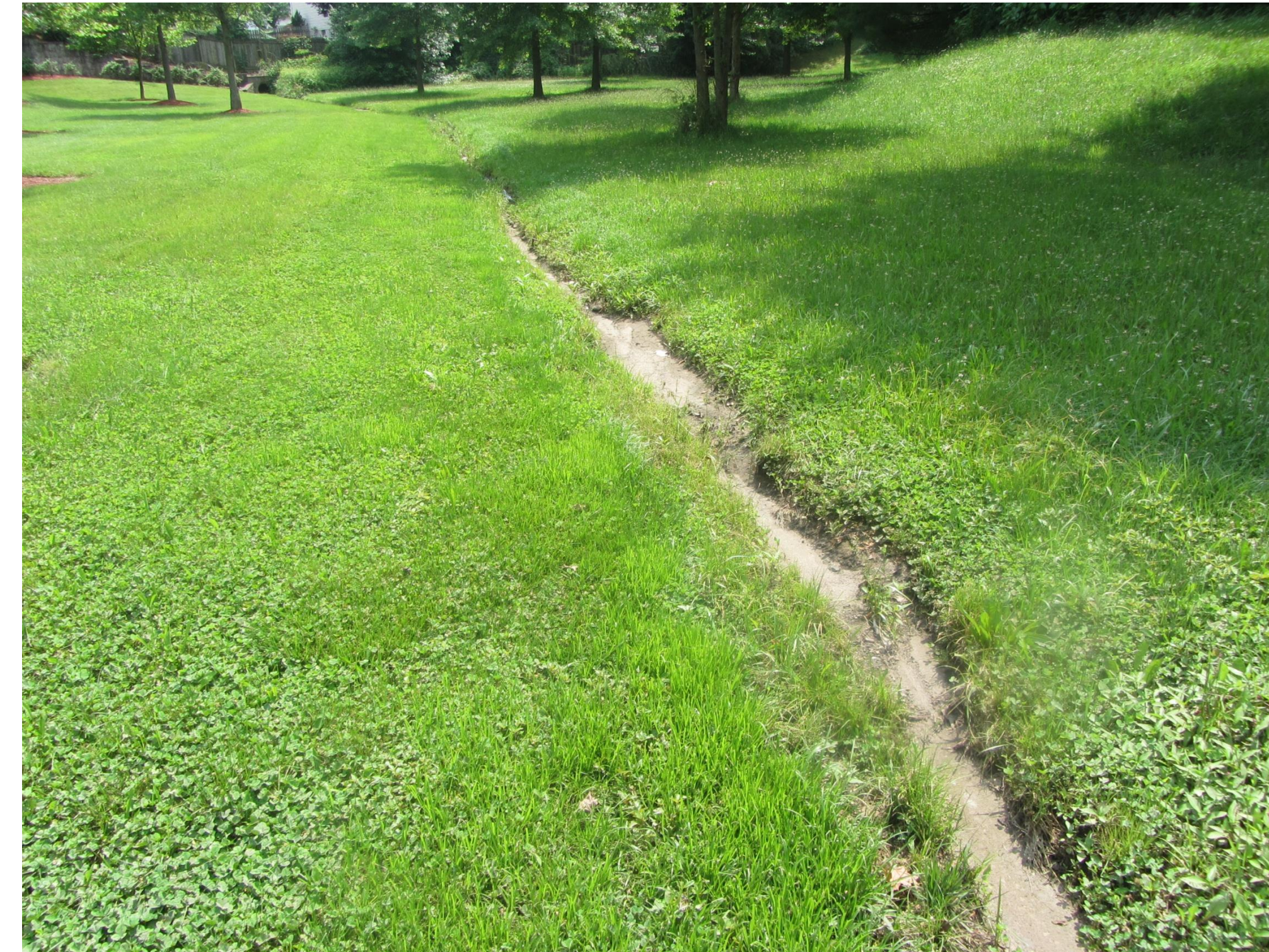
Sediment accumulation in low flow channel
