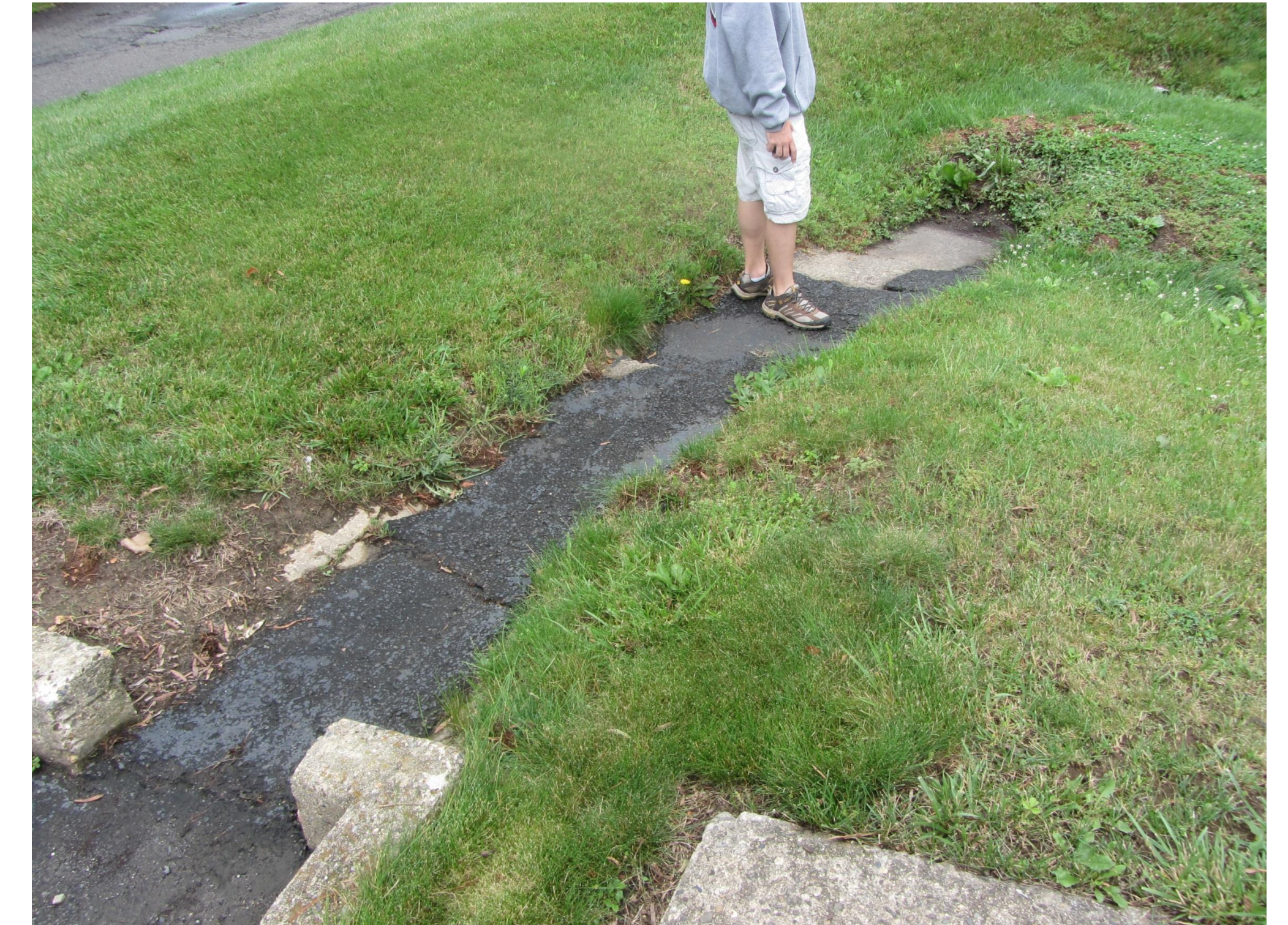
Erosion and breakage at inlet
