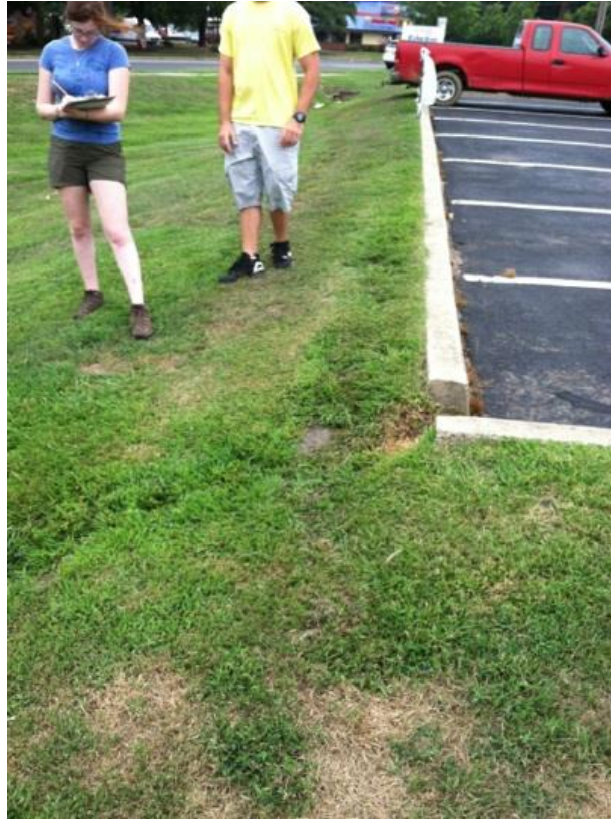
Erosion at inlet
