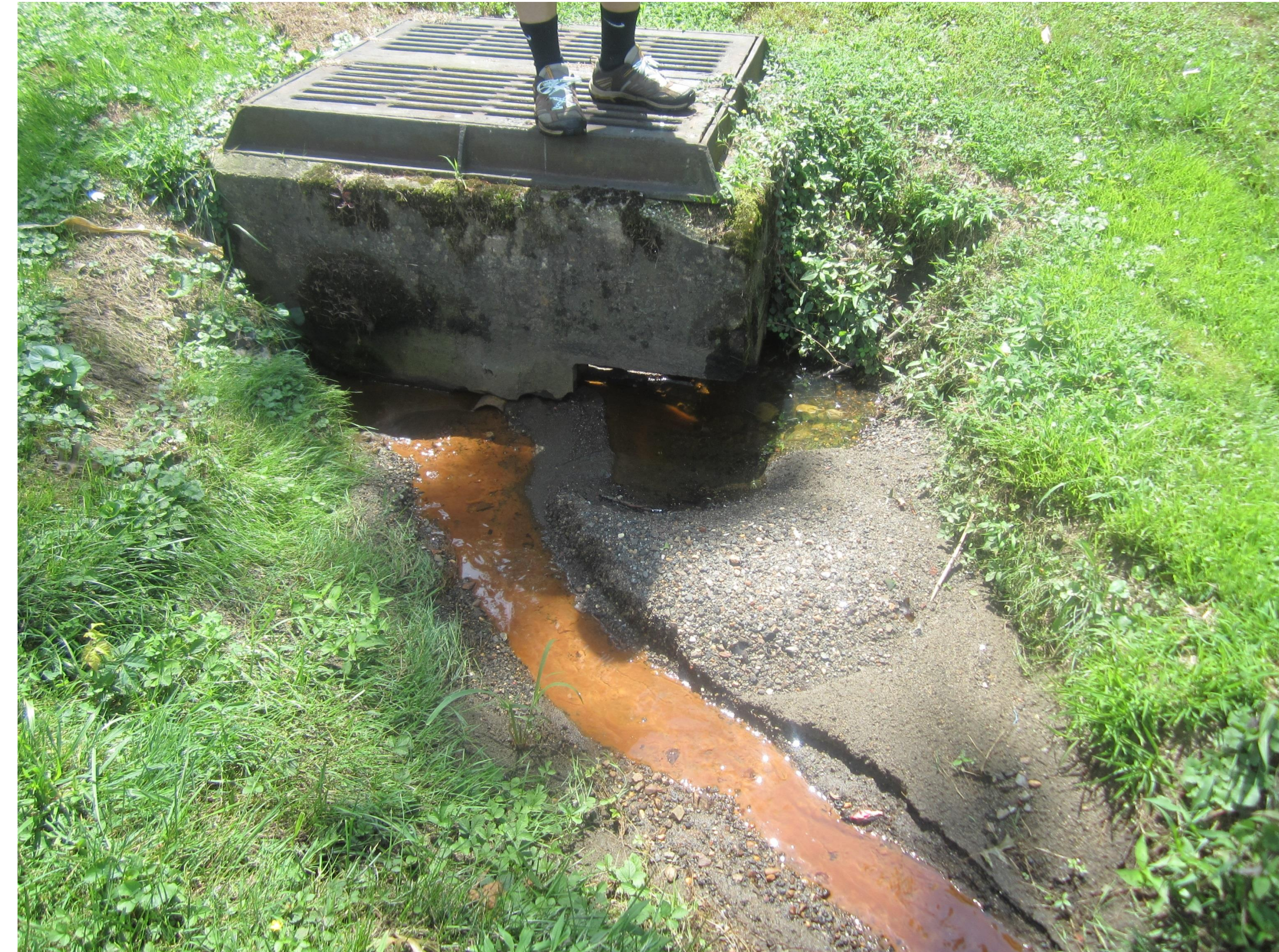
Outlet structure in need of replacement
