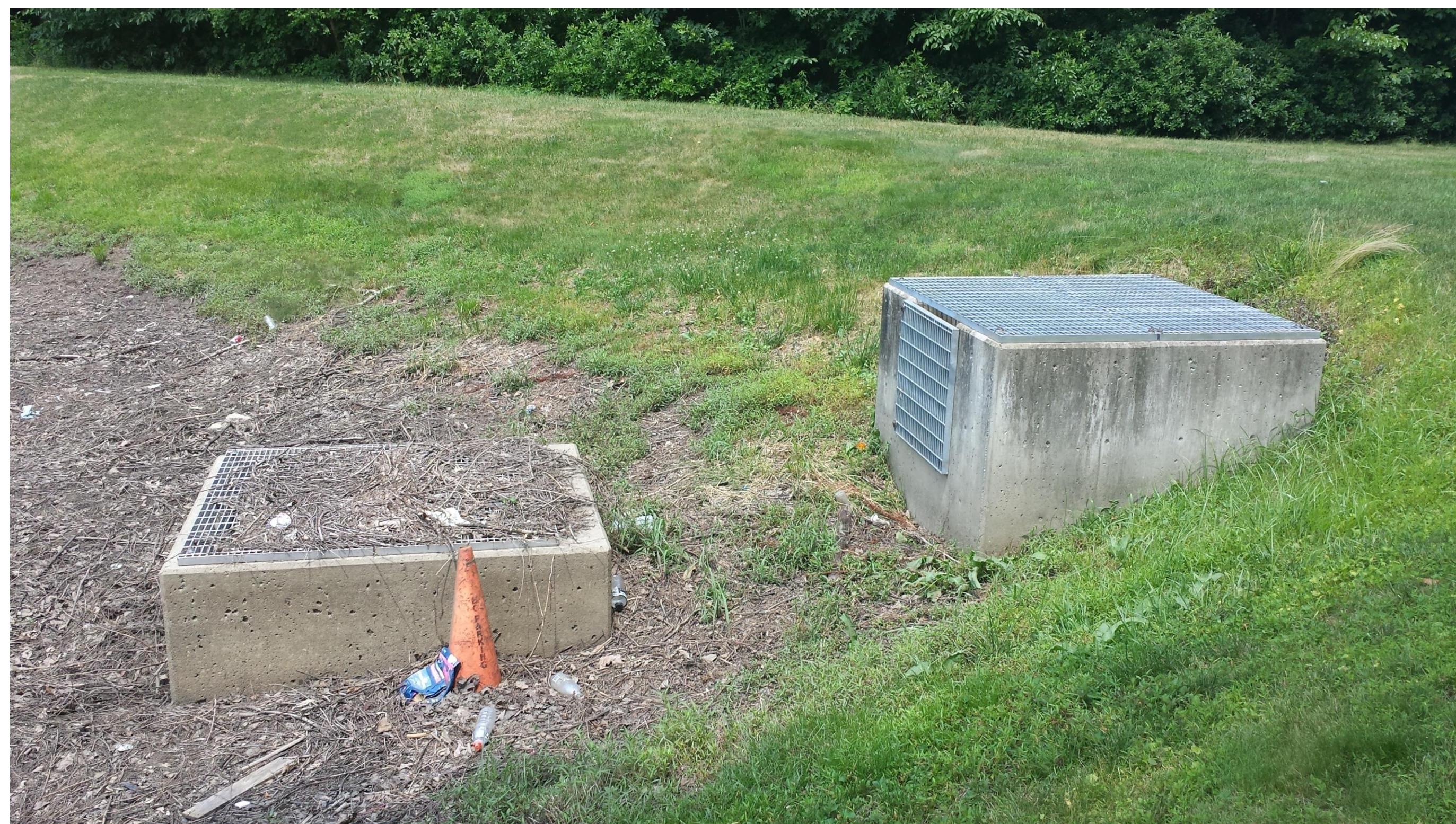
Side view of outlet
