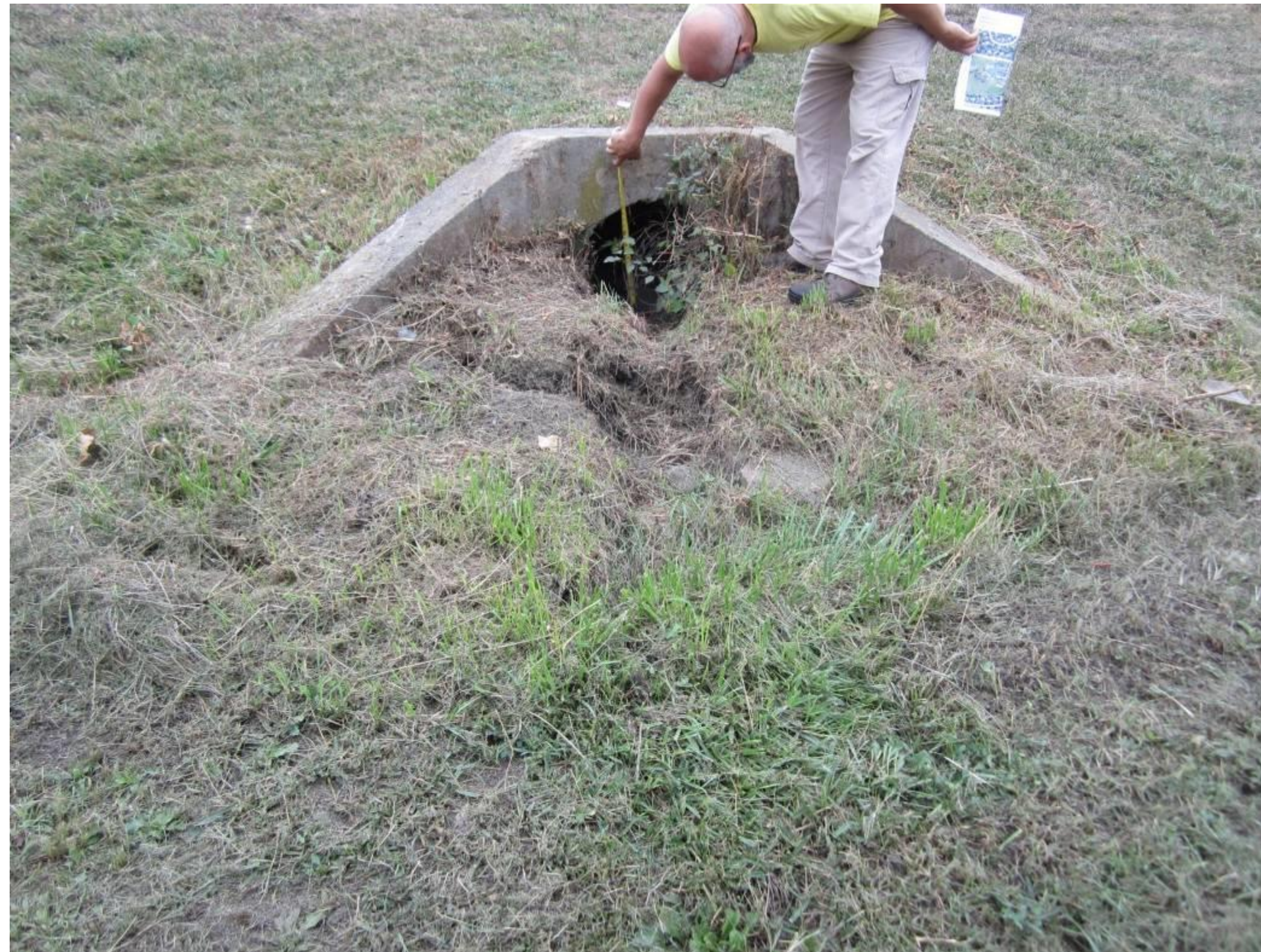
Sediment accumulation in the inlet
