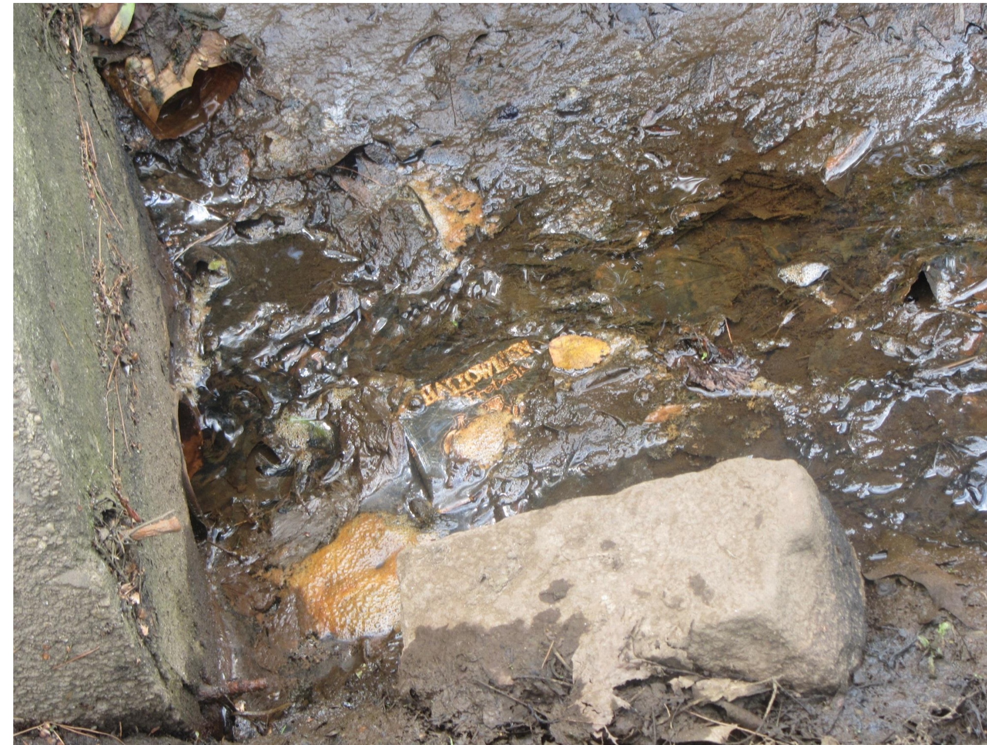
Clogged outlet low flow orifice
