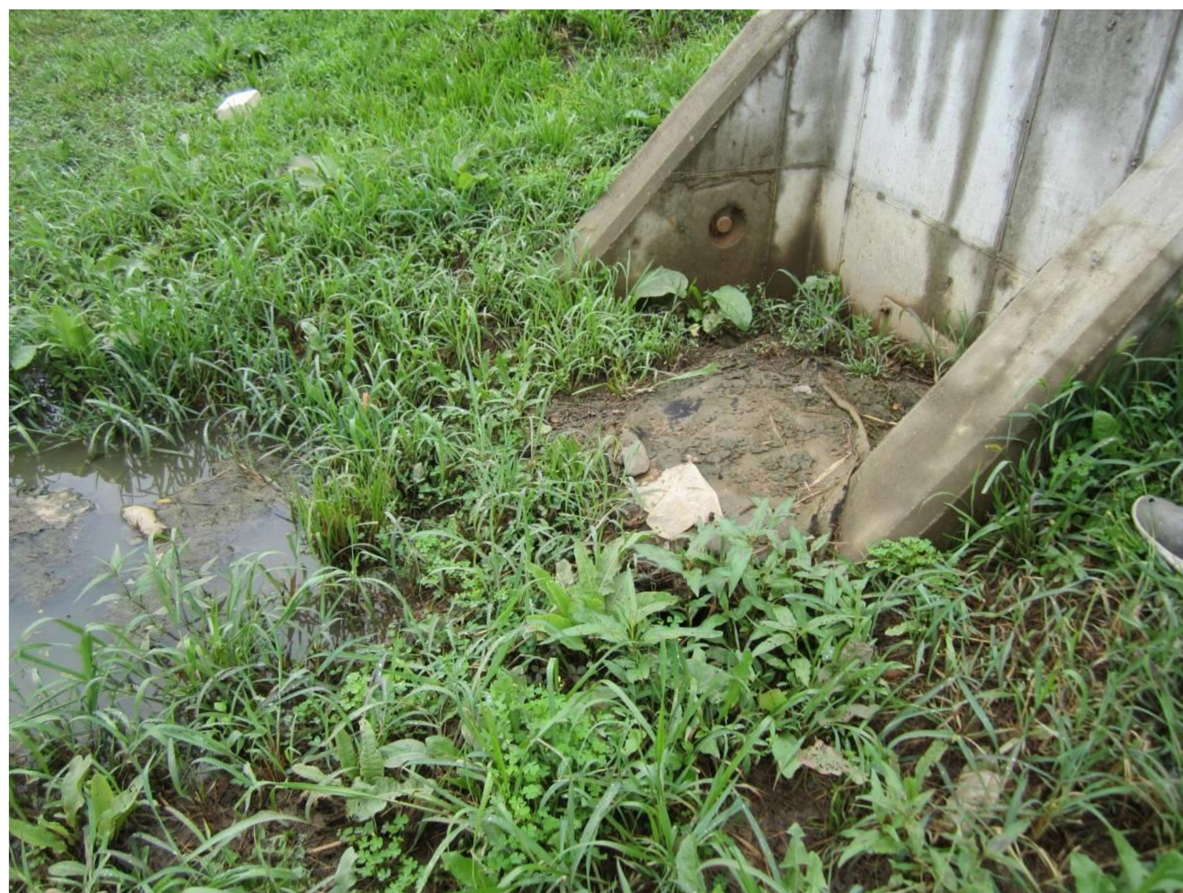
Clogged outlet orifice
