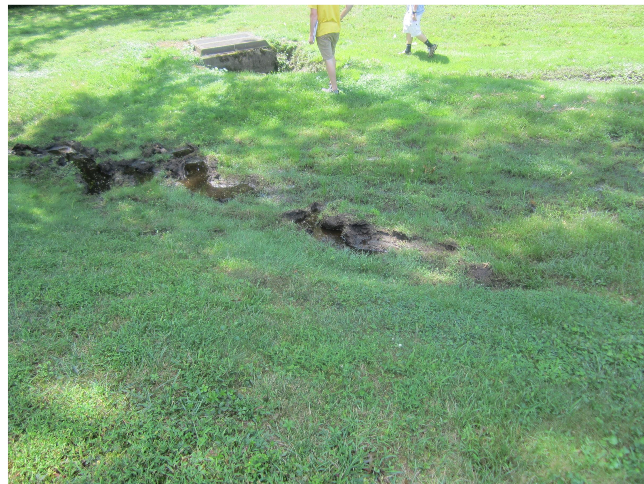
Erosion in basin bottom
