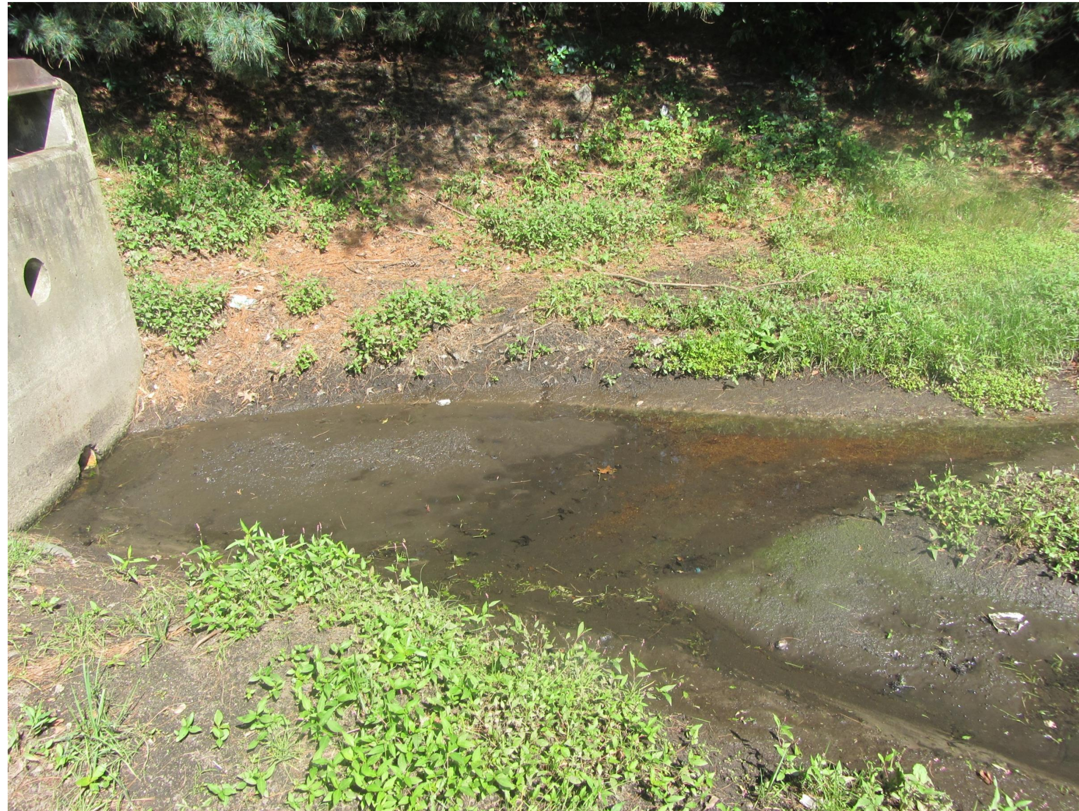
Sediment accumulated in front of outlet
