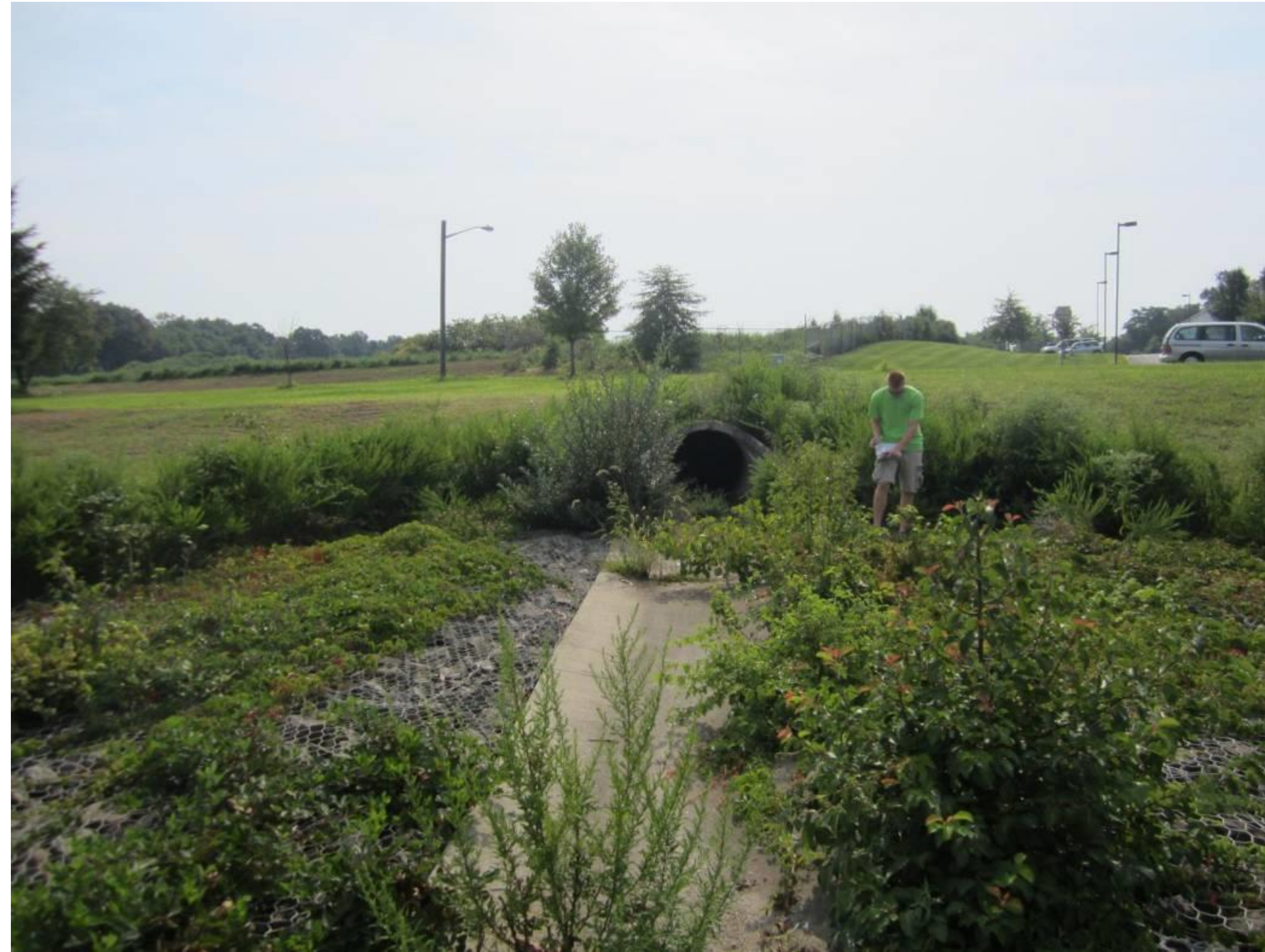
Inlet and rip rap protection
