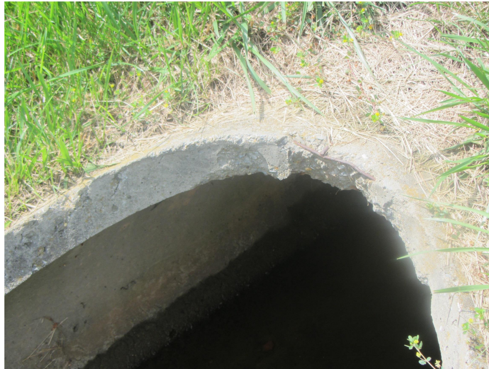
Concrete deterioration on eastern inlet
