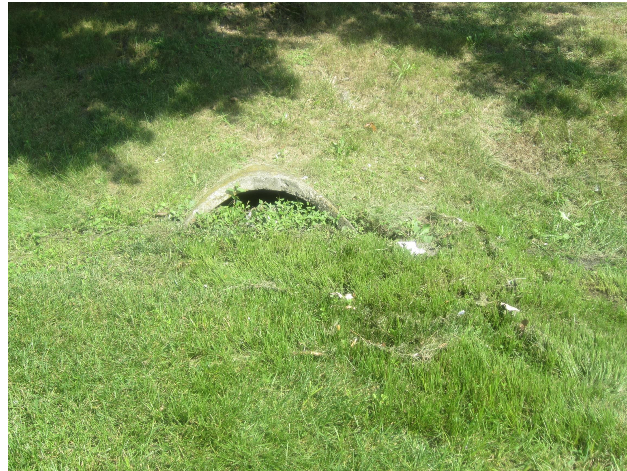
Inlet filled with sediment
