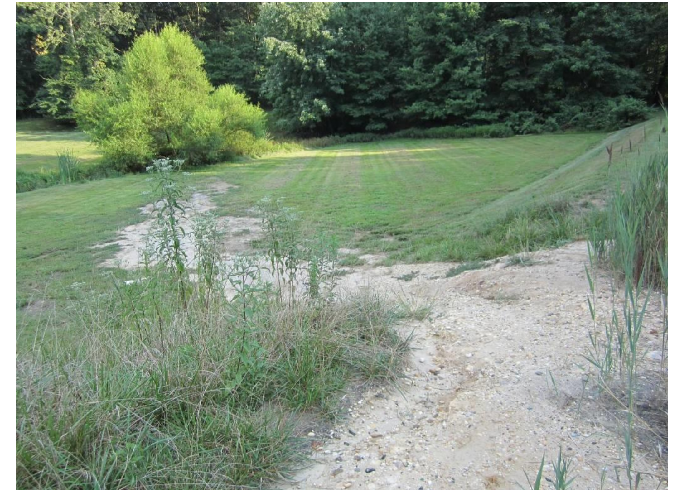
Slumping/failing basin embankment
