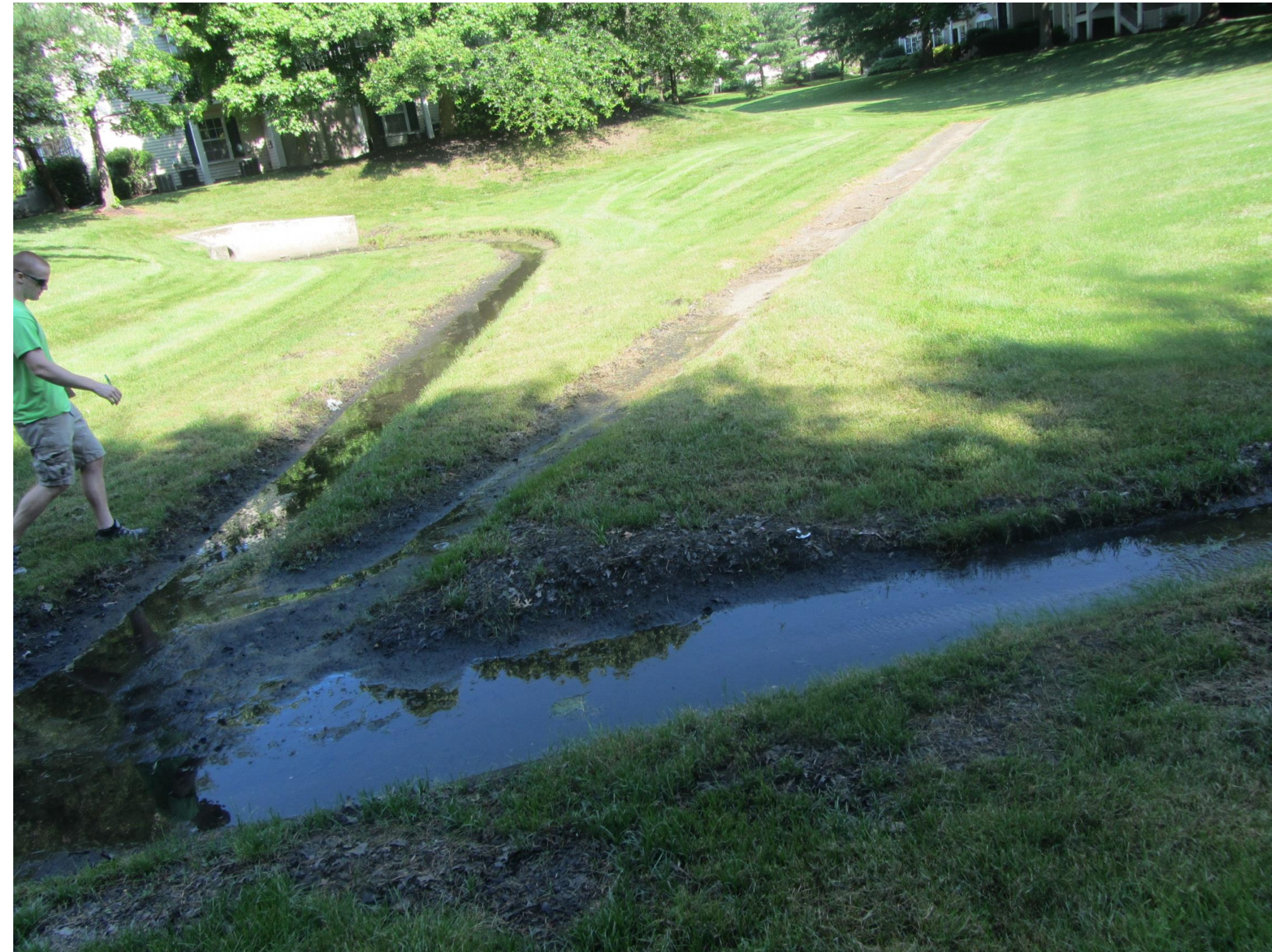
Excess sediment in low flow channels
