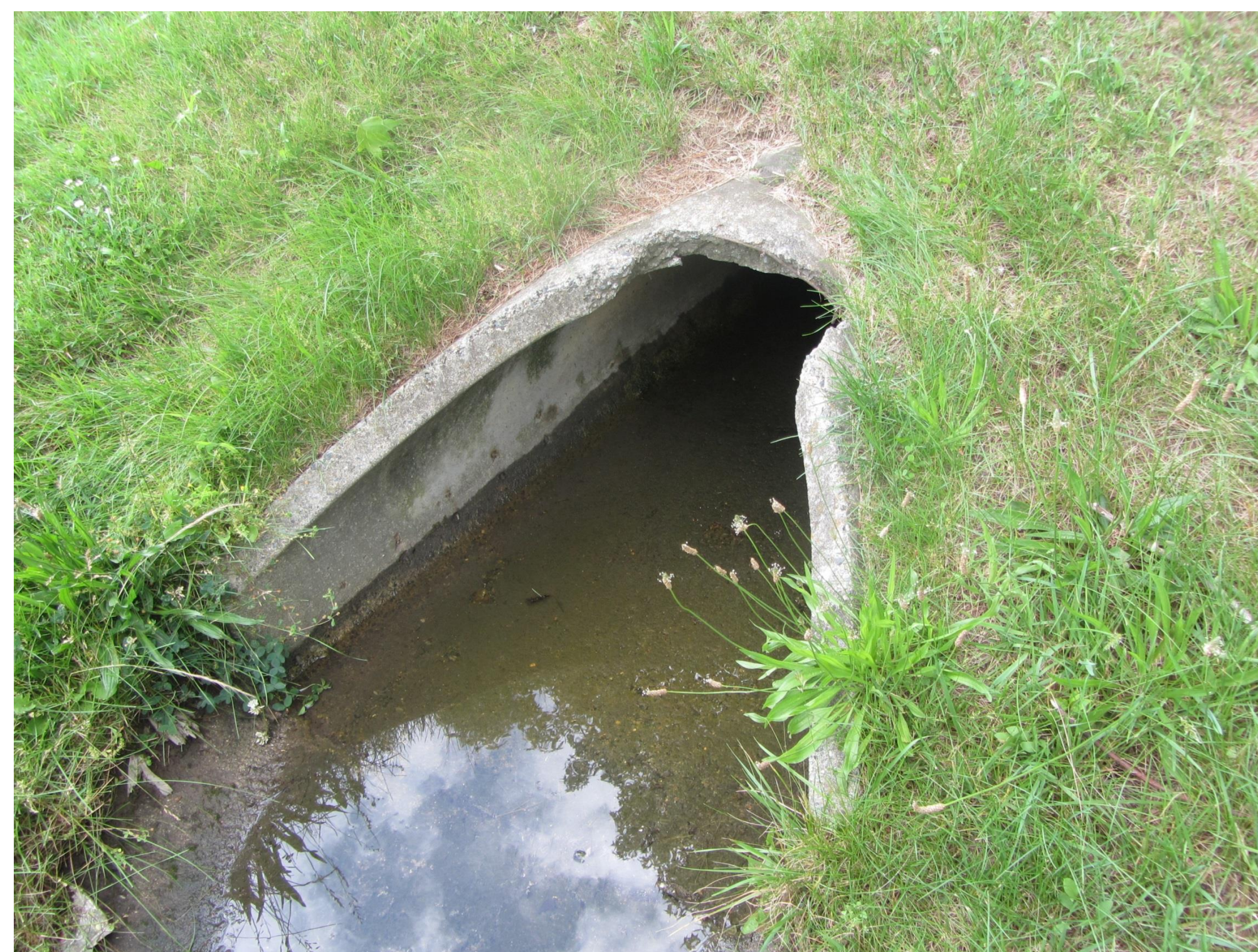
Breakage on northeastern inlet
