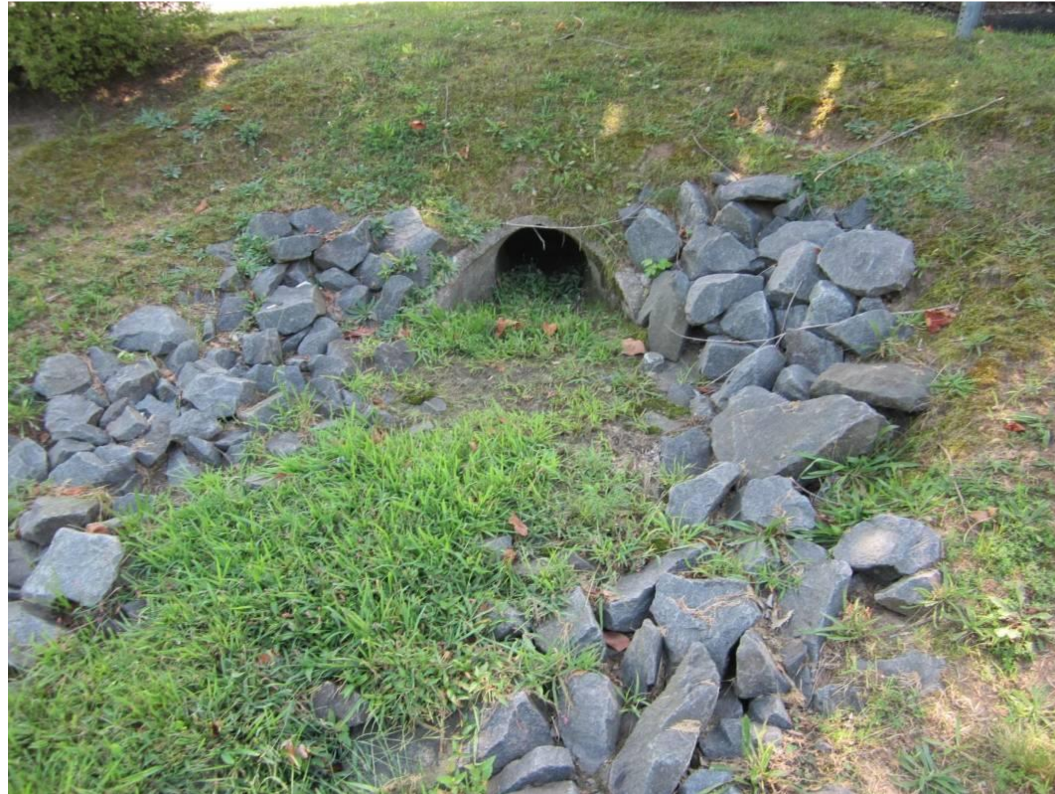
Inlet with sediment accumulation
