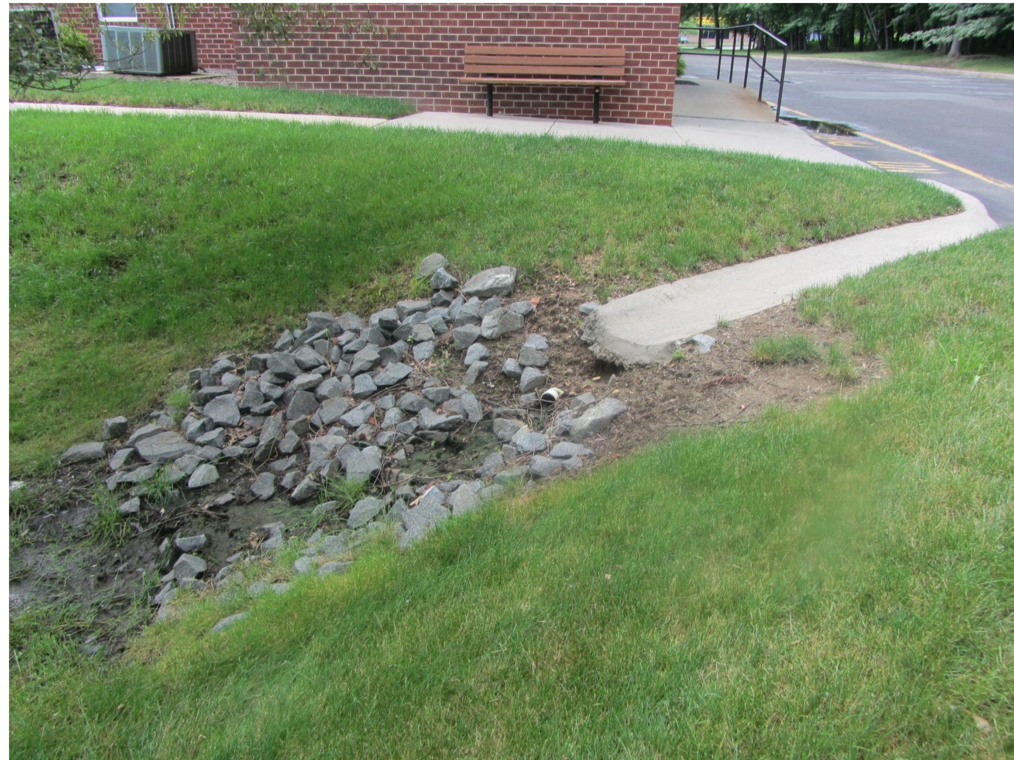
Erosion around northeastern inlet
