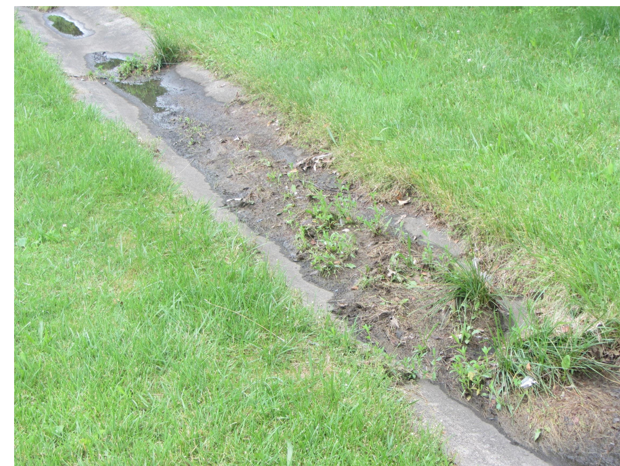
Excess sediment in low flow channel
