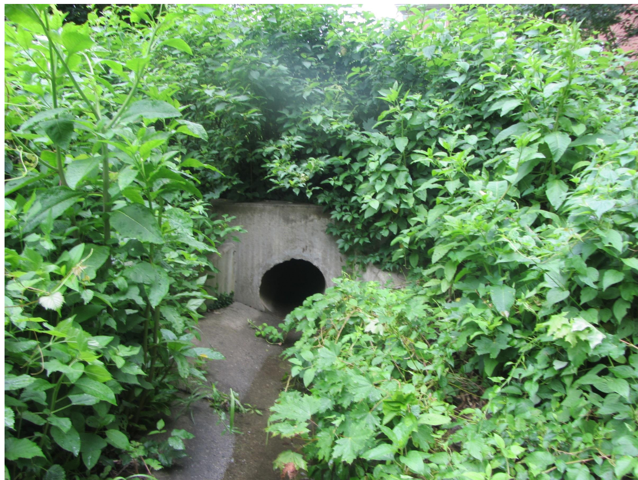
Plant growth around inlet
