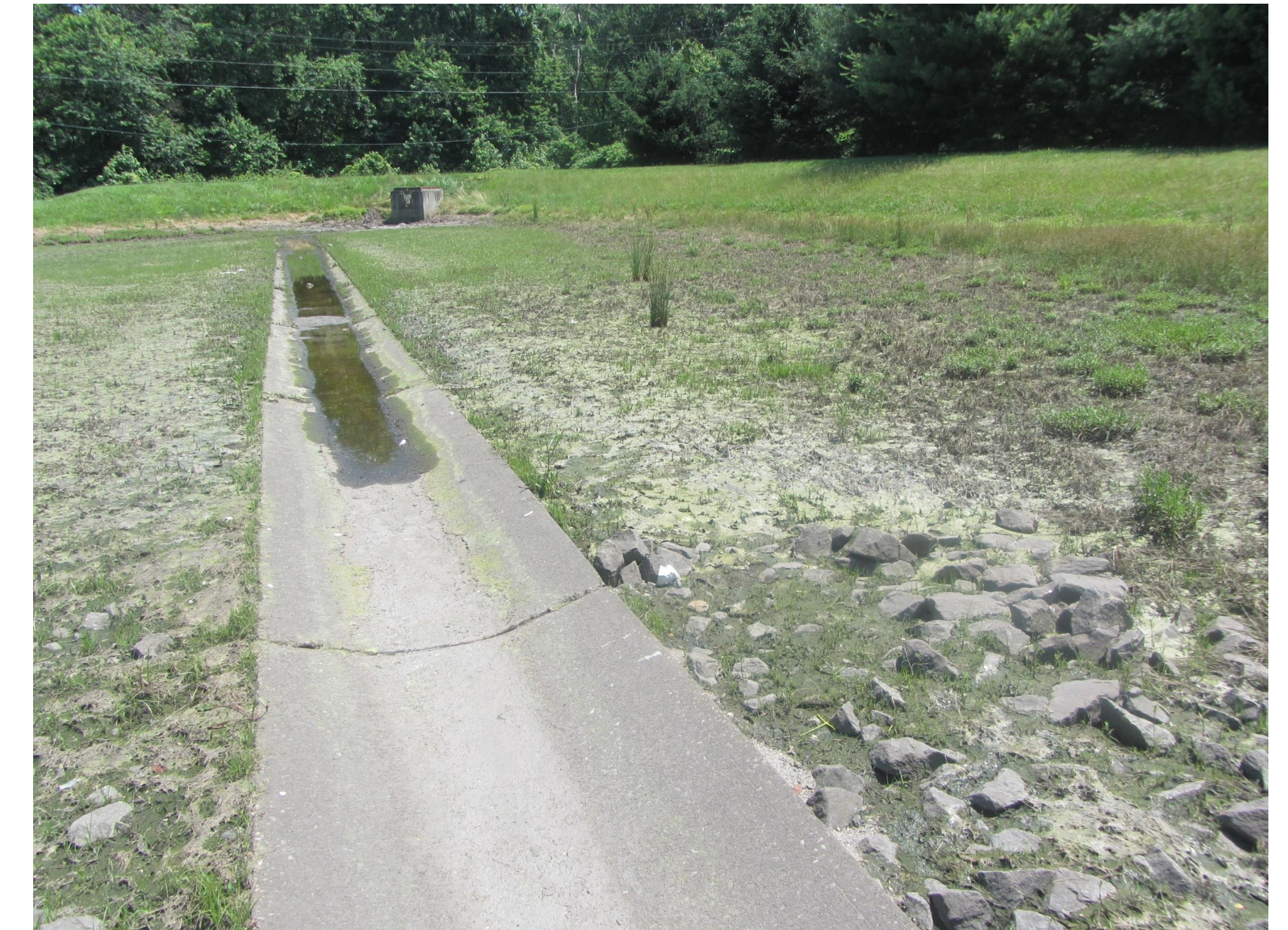
Exposed earth alongside low flow channel
