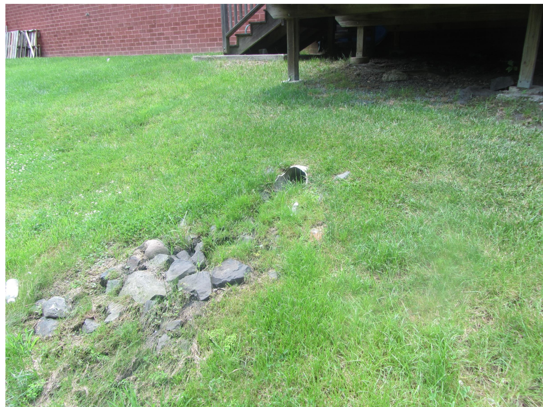
Erosion in front of inlet
