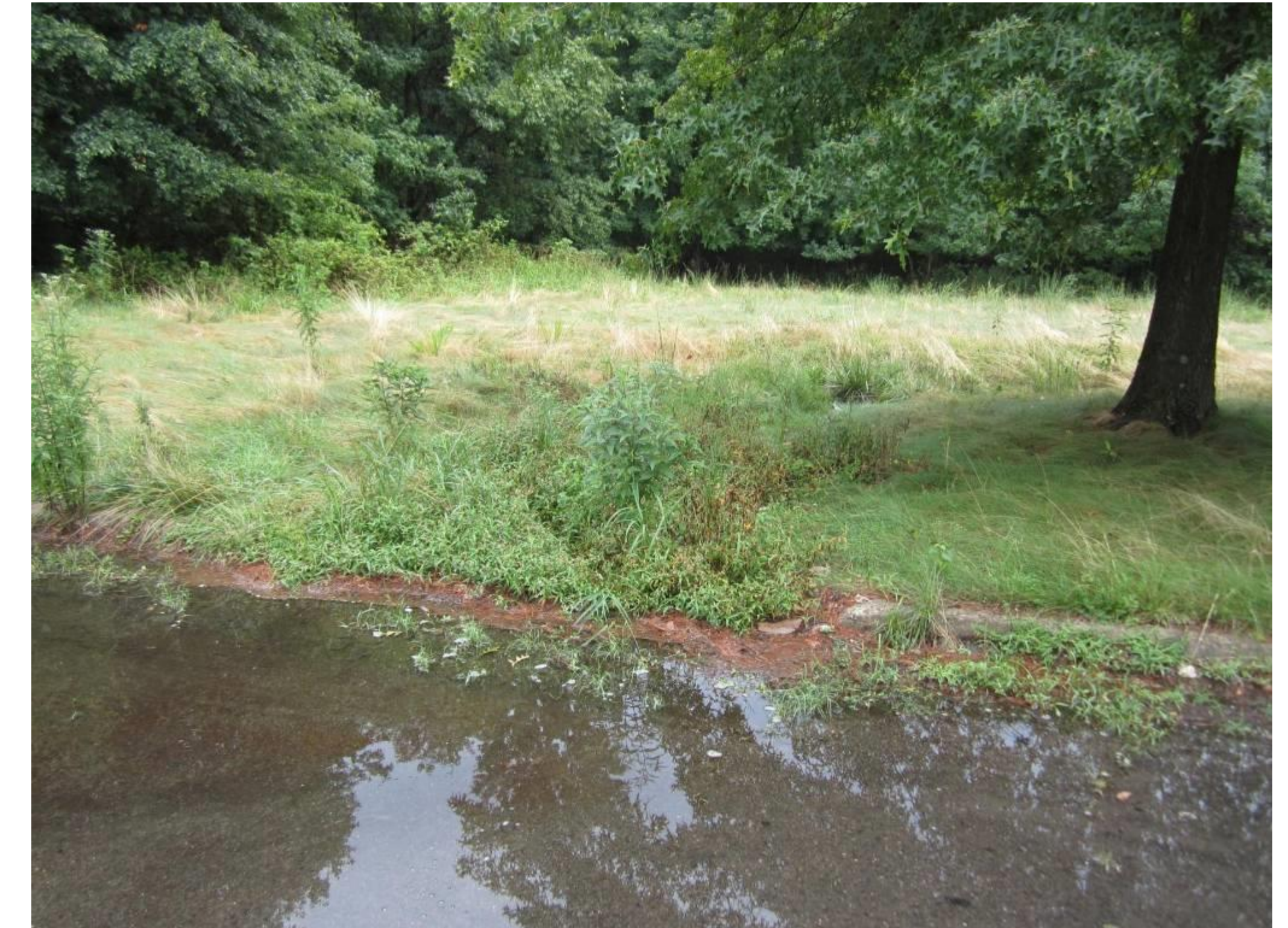
Clogged curb cut, ponding
