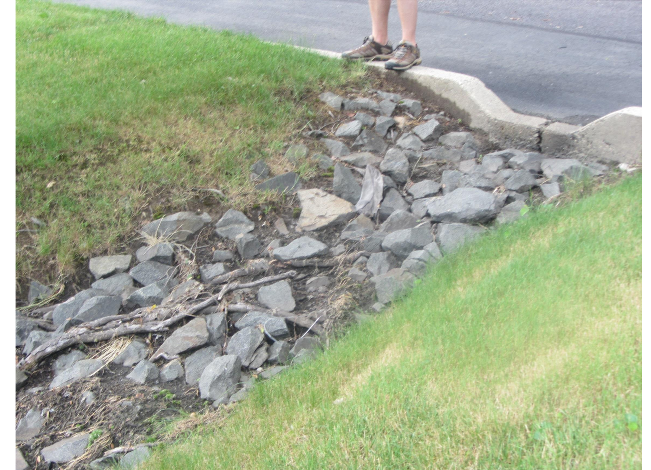
Erosion around southeastern inlet
