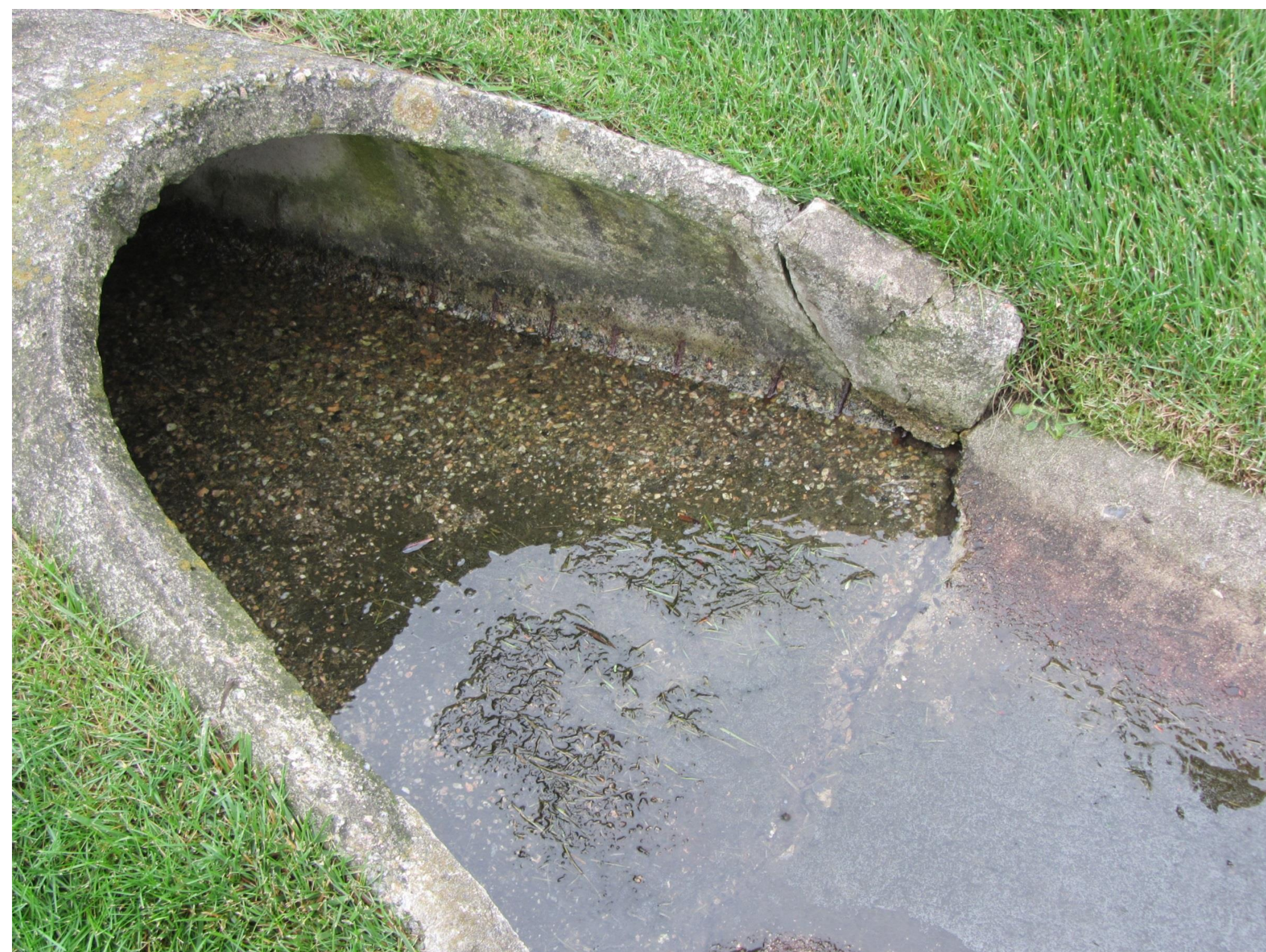
Inlet structure breakage
