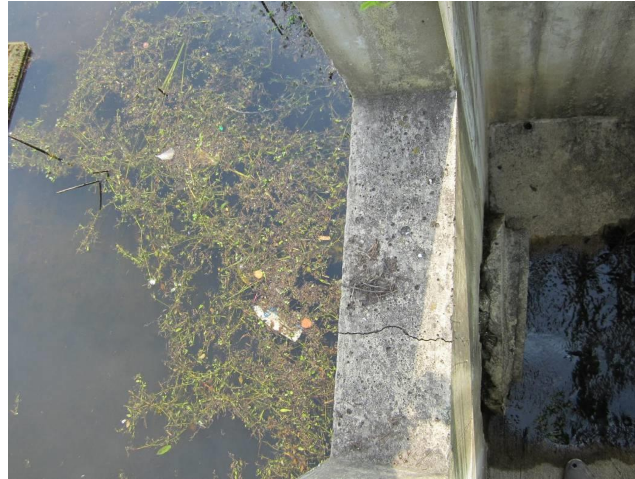
Clogged outlet structure
