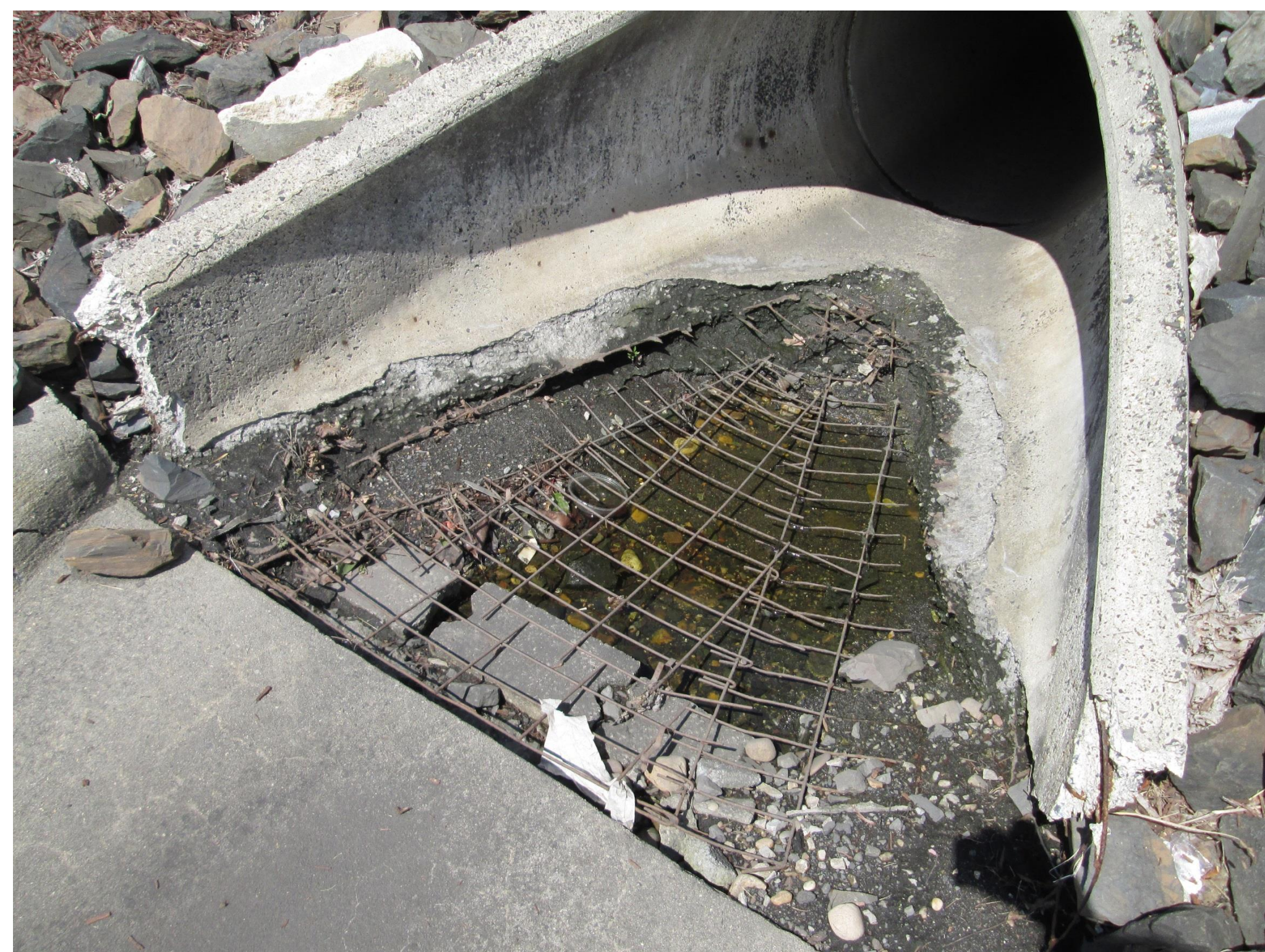
Erosion of inlet
