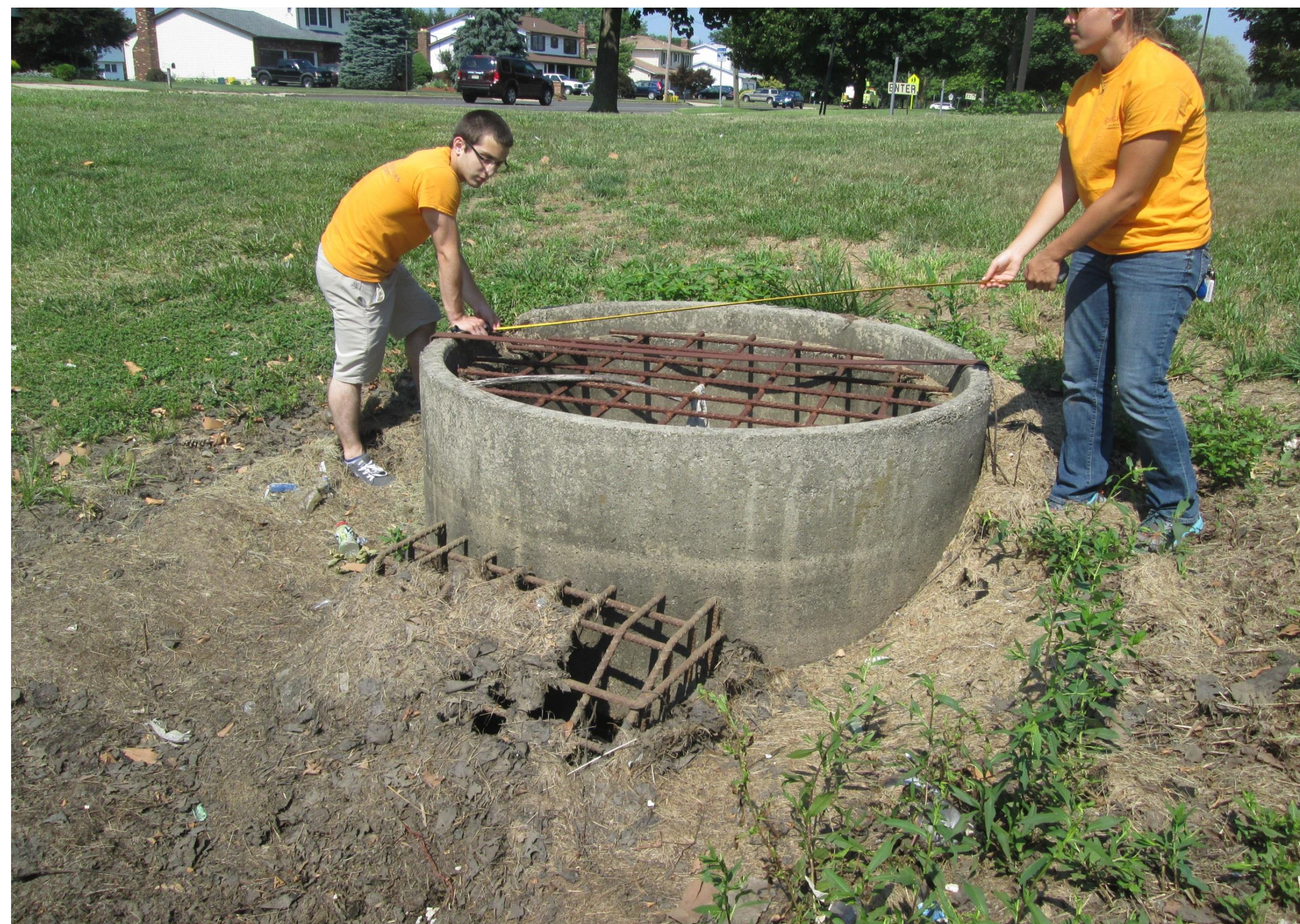
Degraded outlet structure
