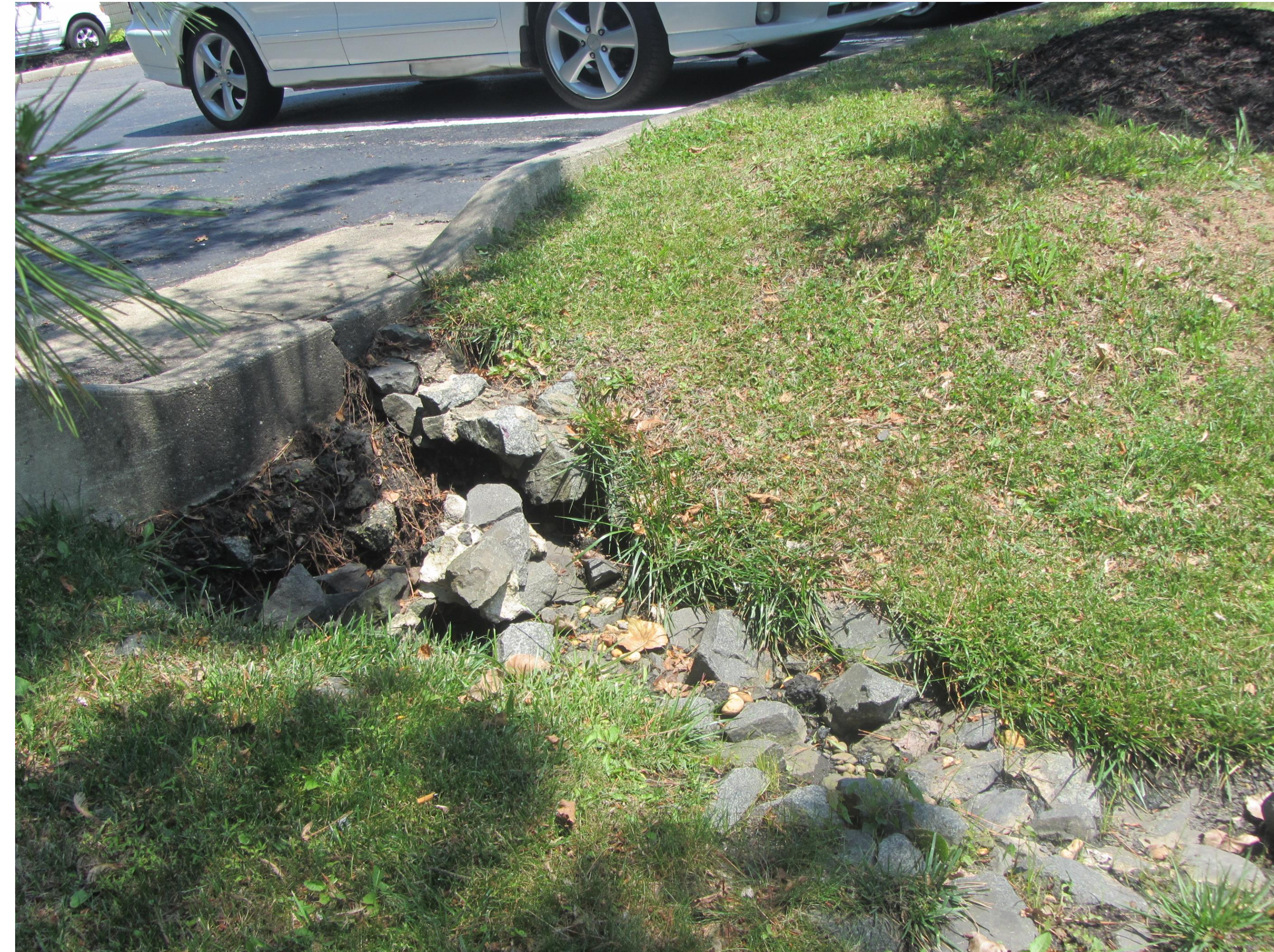
Erosion at curb cut inlet
