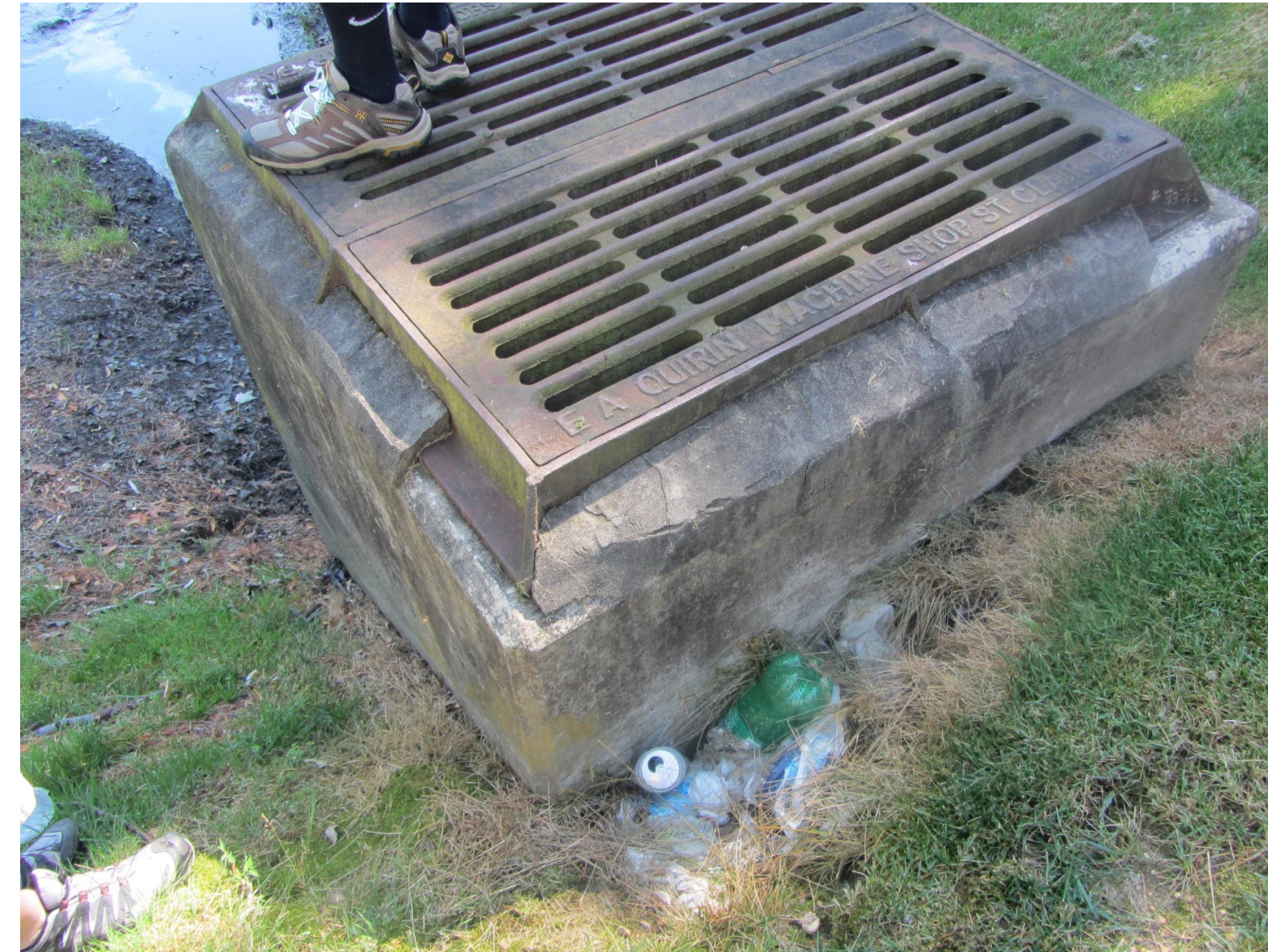
Slumping behind outlet structure
