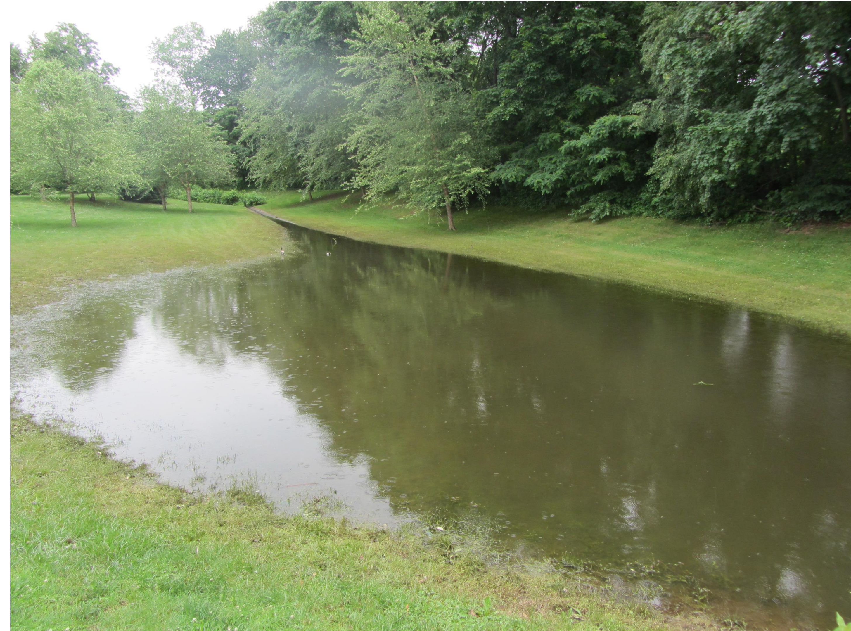
Severe ponding in basin
