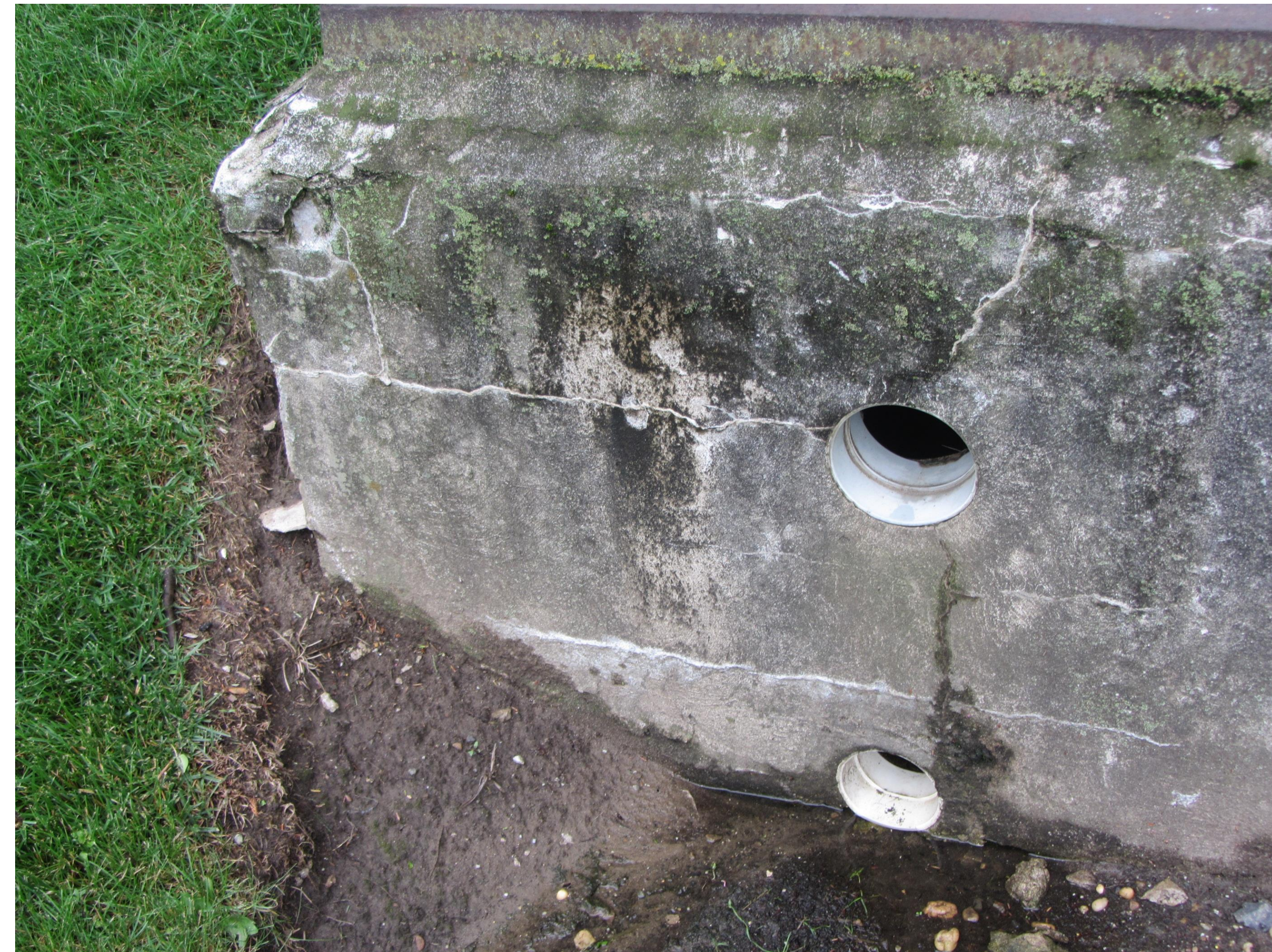
Outlet structure with slumping and breakage
