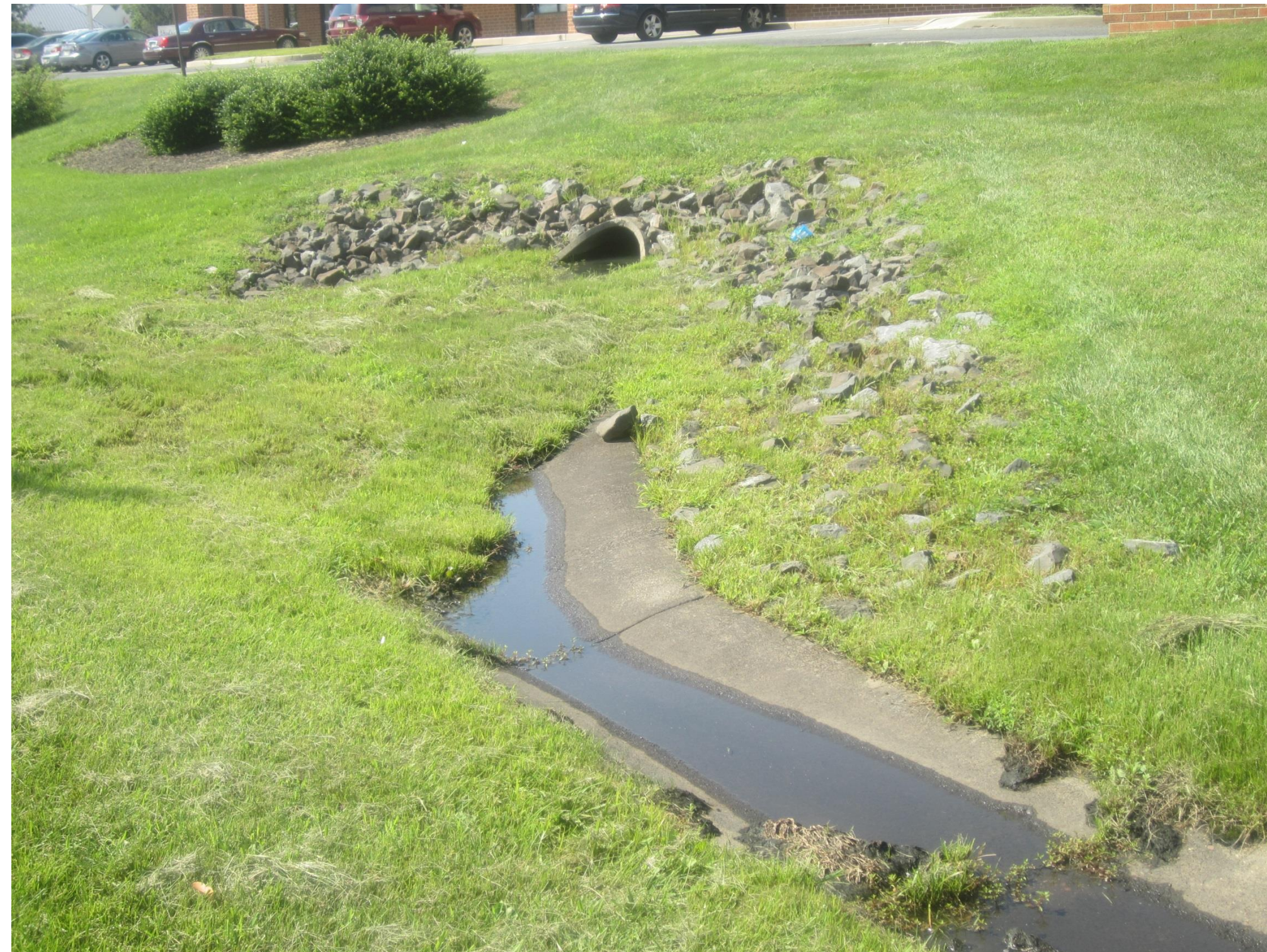
Inlet and low flow covered in sediment
