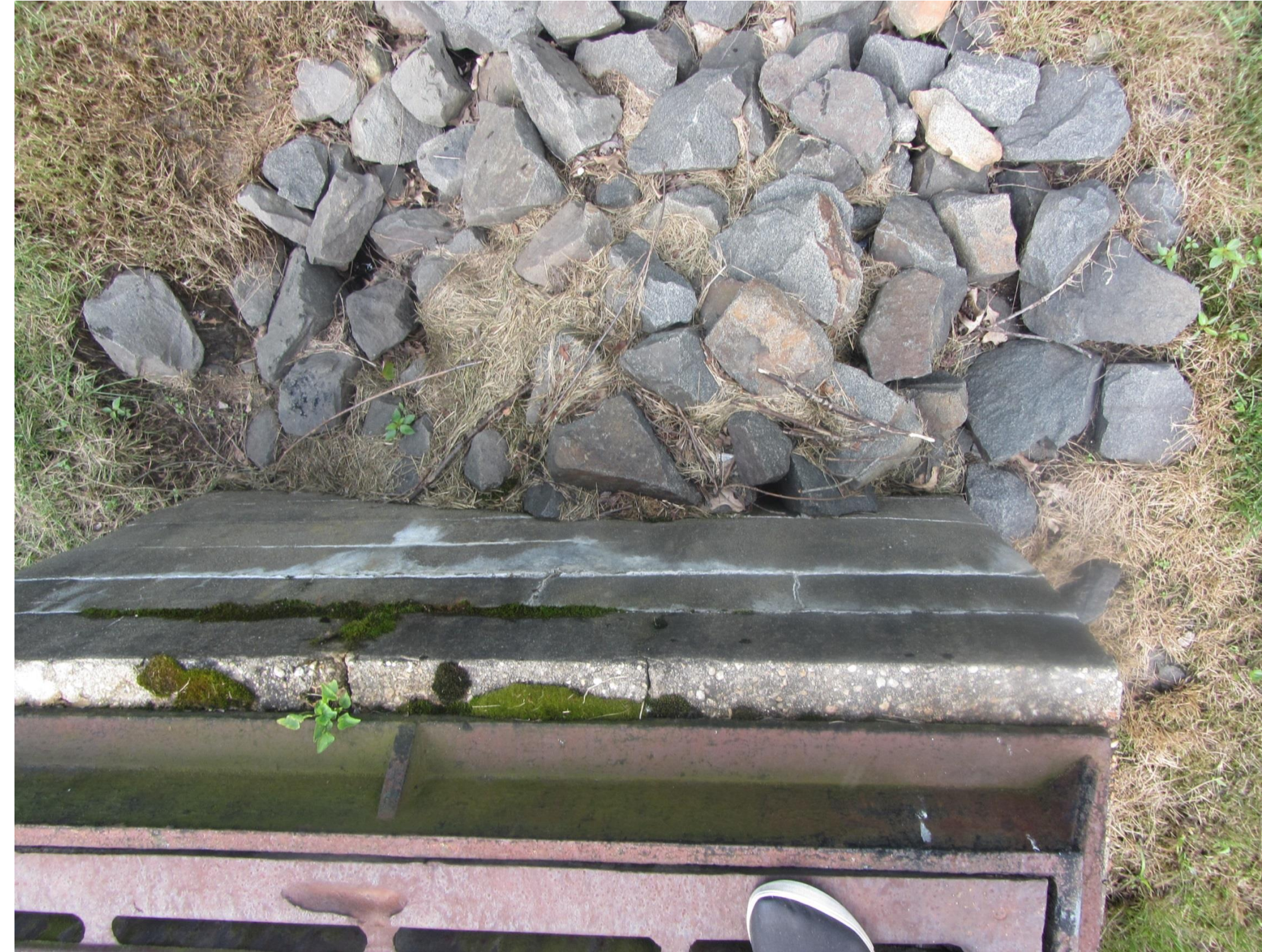
Rip-rap blocking low flow orifice
