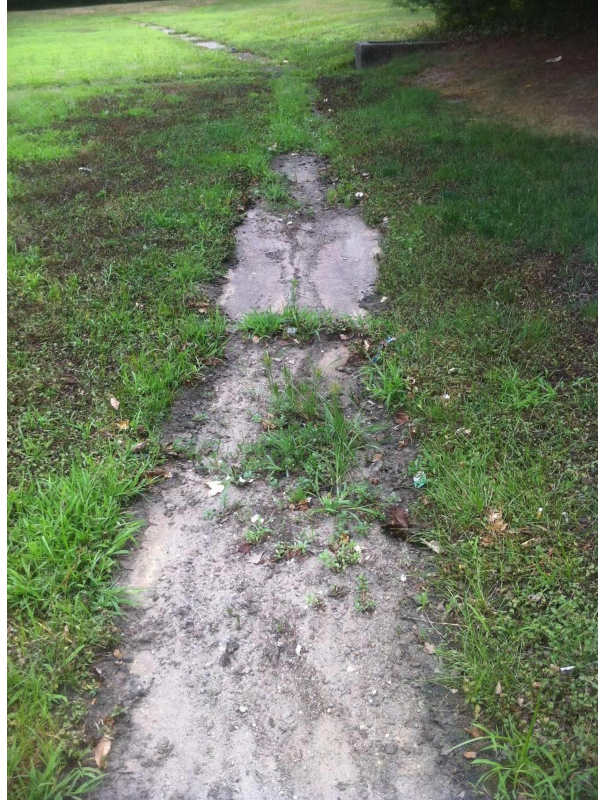
Sediment in low flow channel
