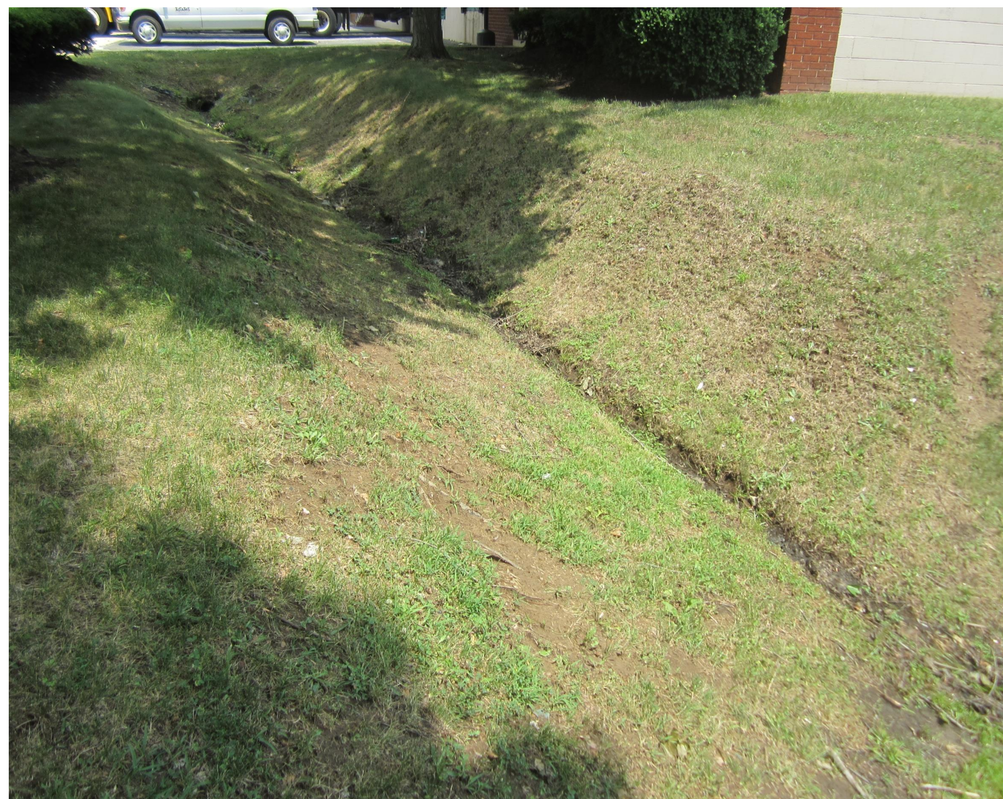
Eroded swale bottom
