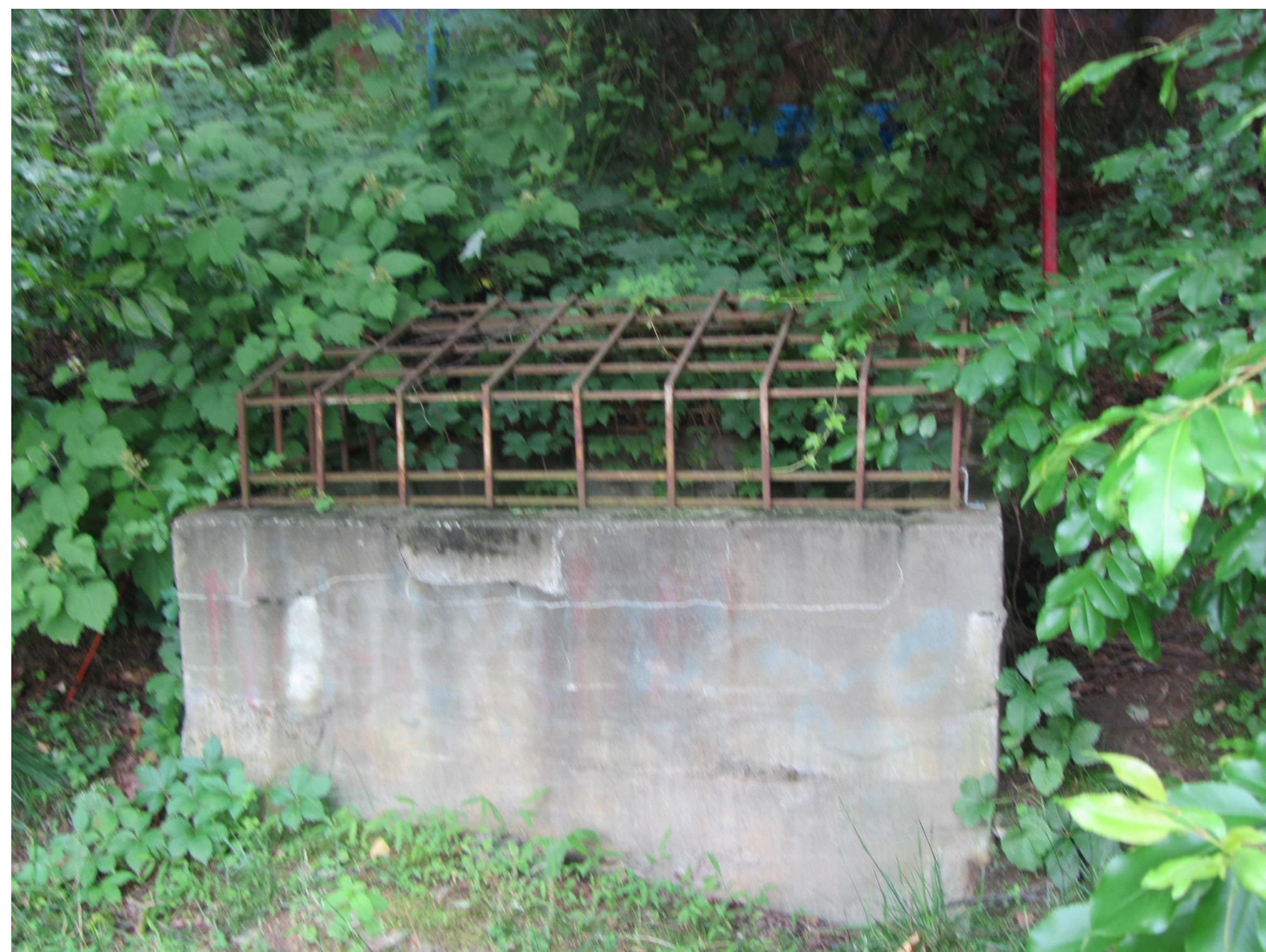
Excessive growth around outlet structure
