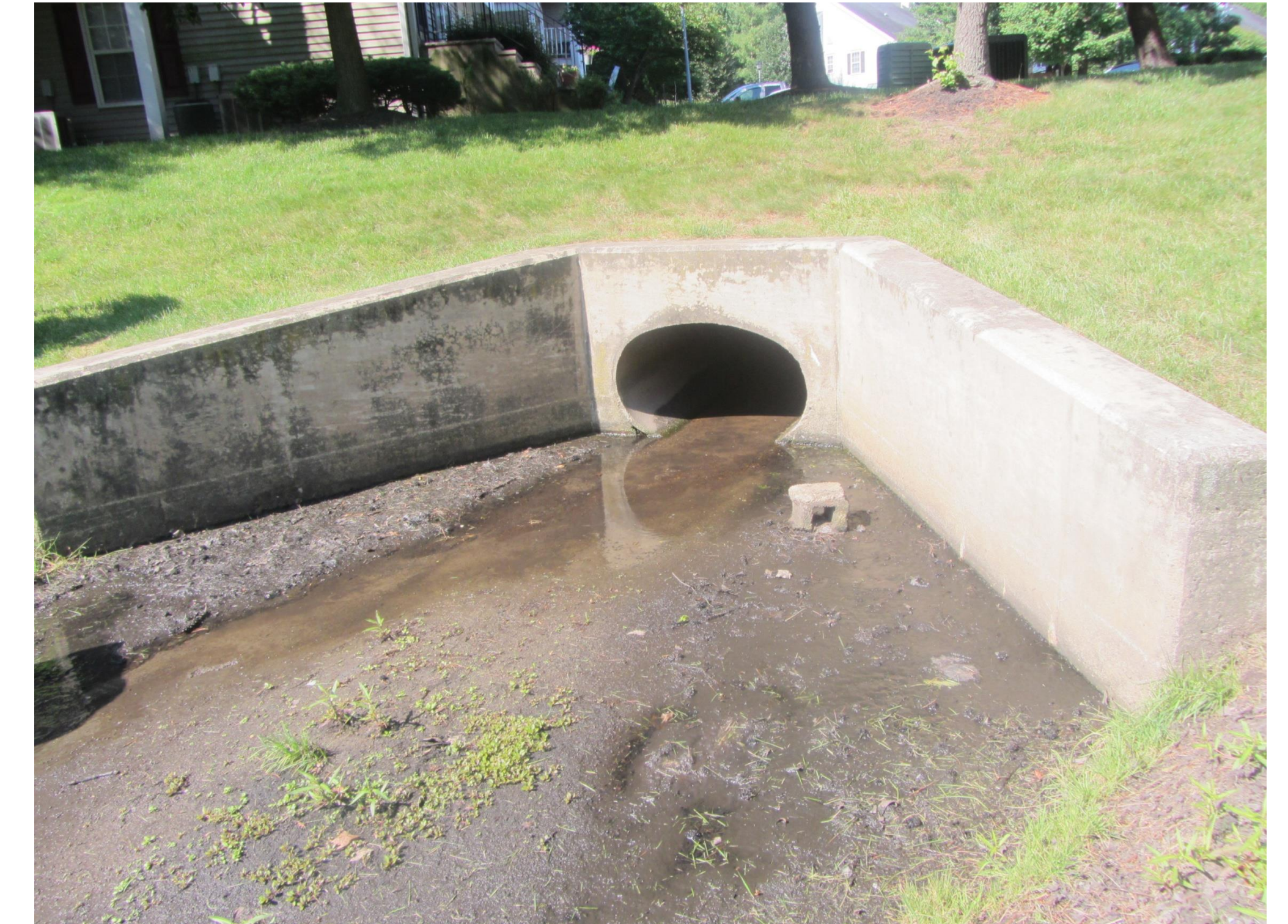
Sediment accumulated in front of inlet
