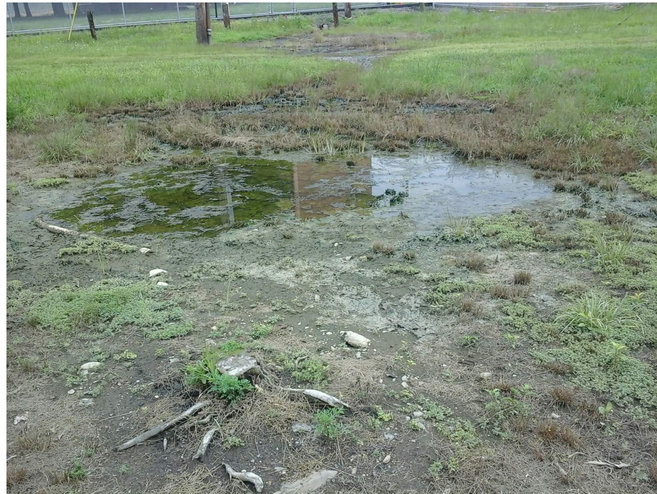
Overview of basin
