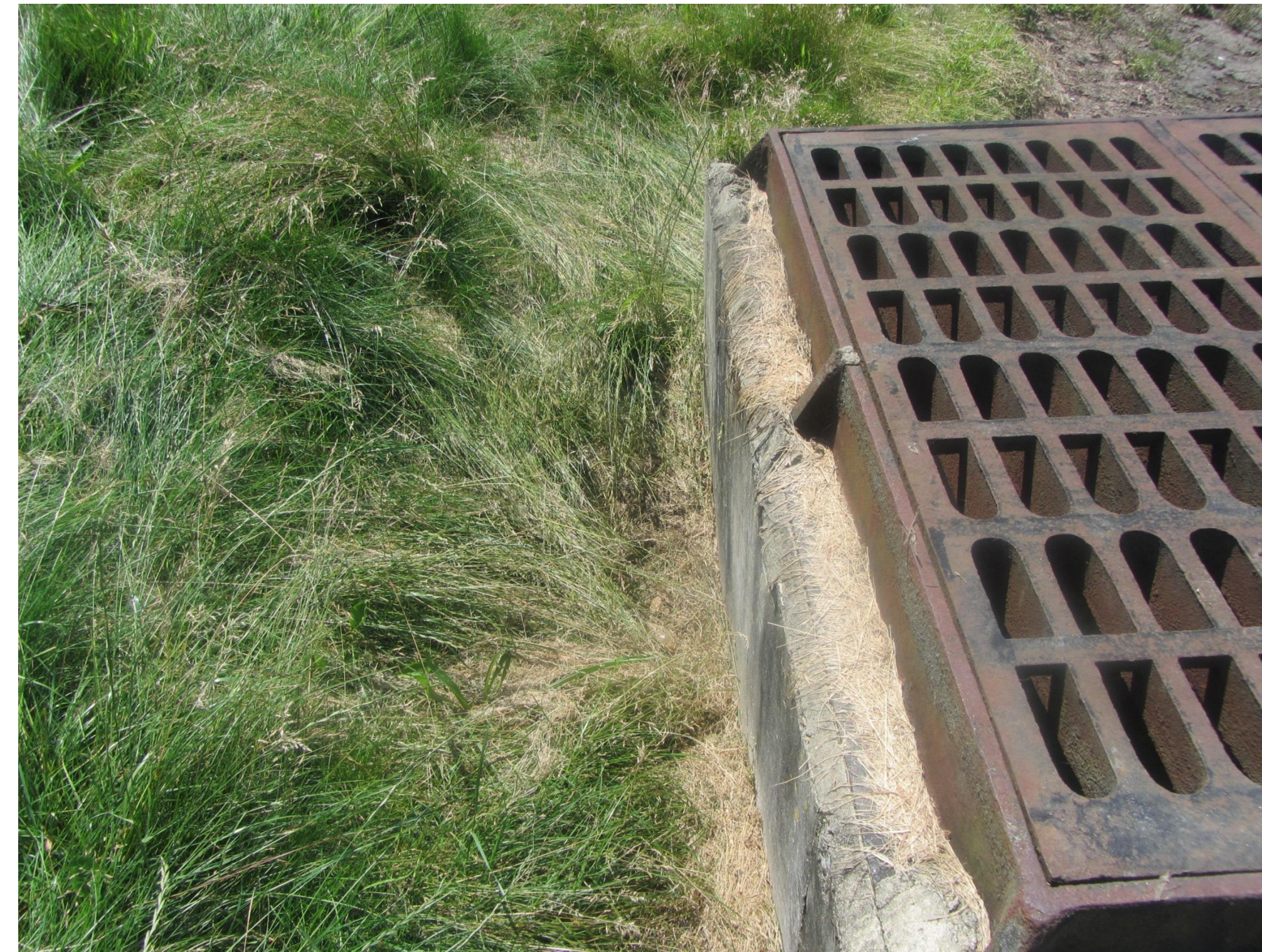
Slumping behind outlet
