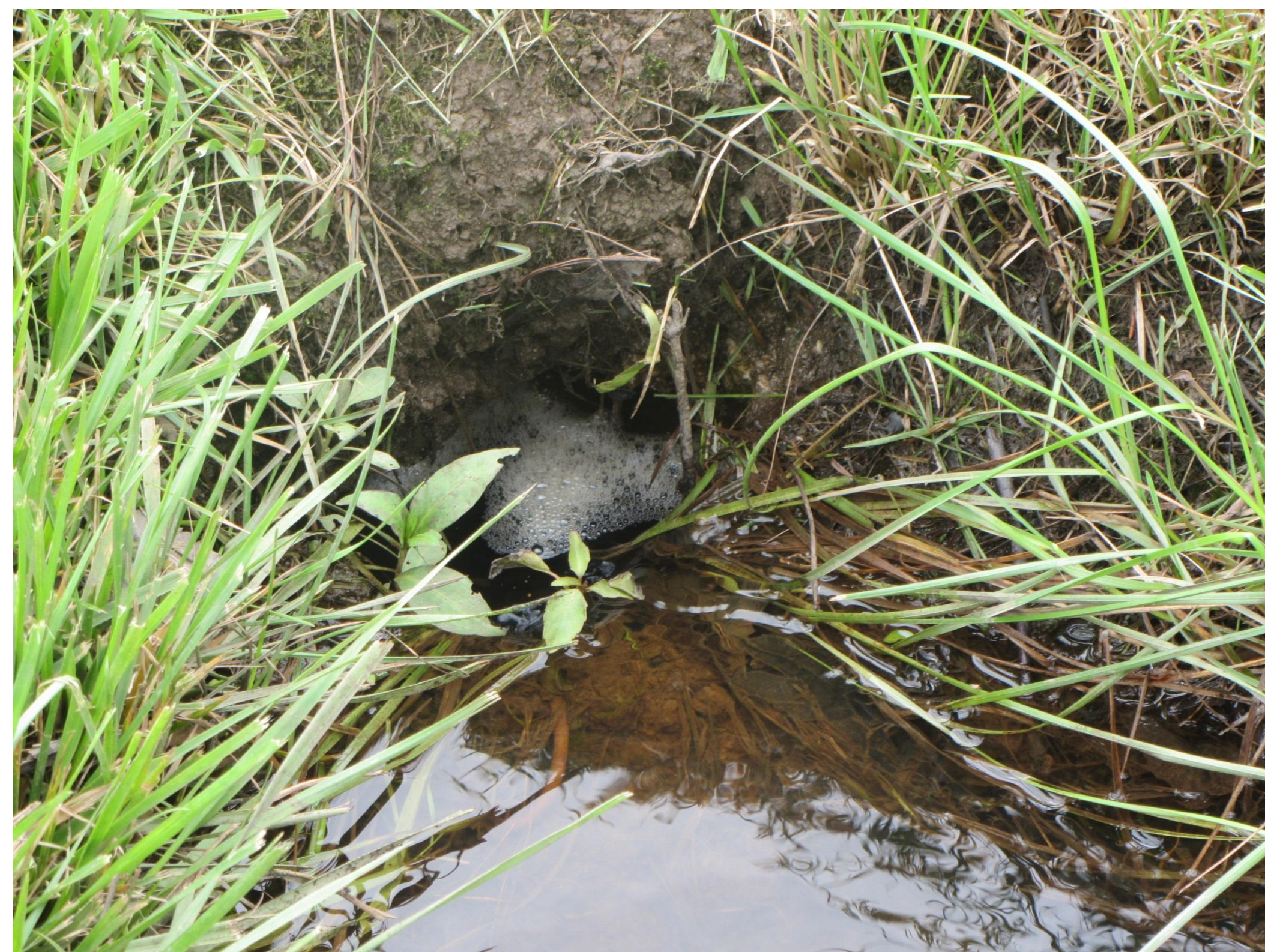
Water exiting through hole
