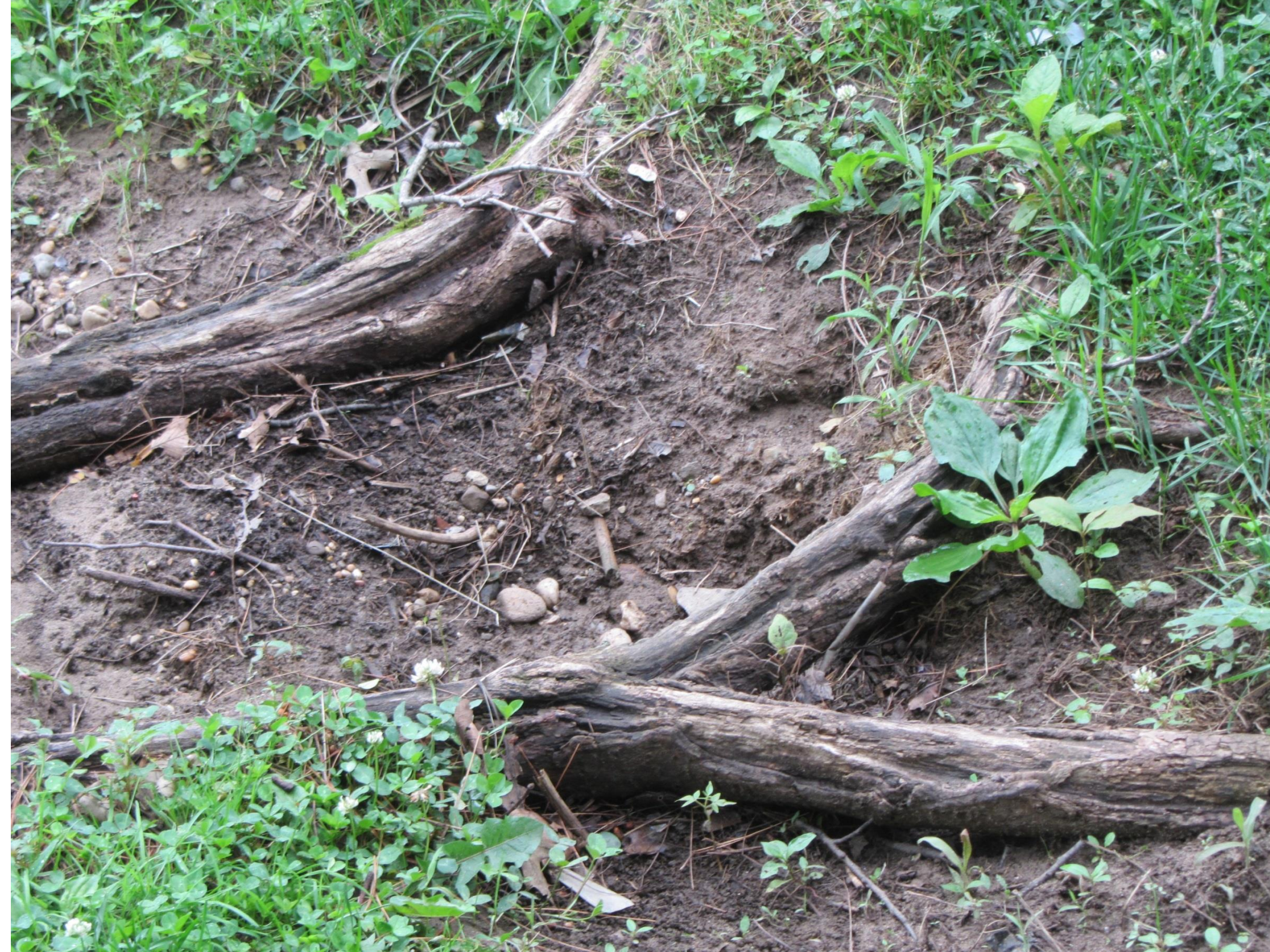
Severe erosion in swale inlet
