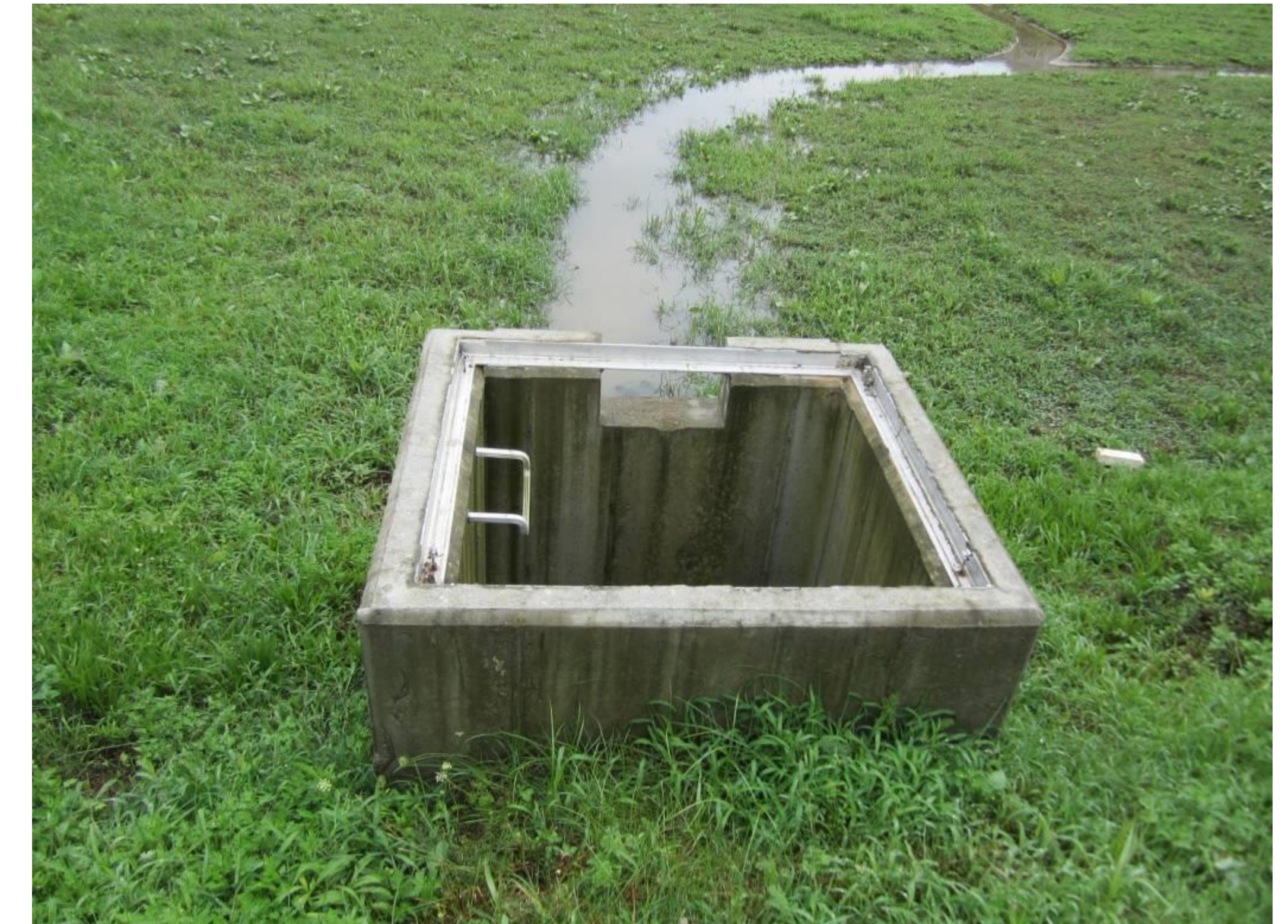
Outlet structure missing grate
