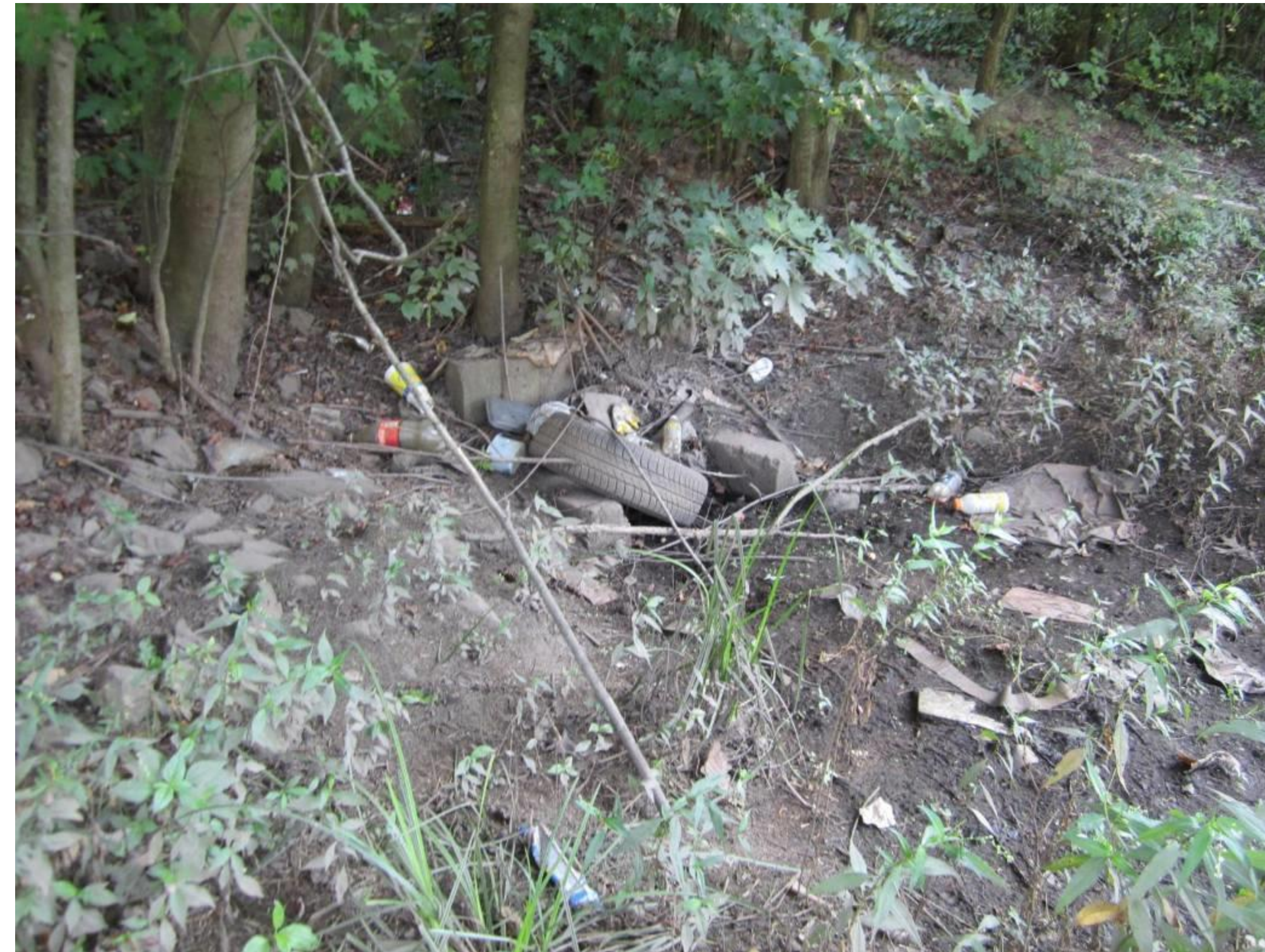
Outlet structure obstructed with litter
