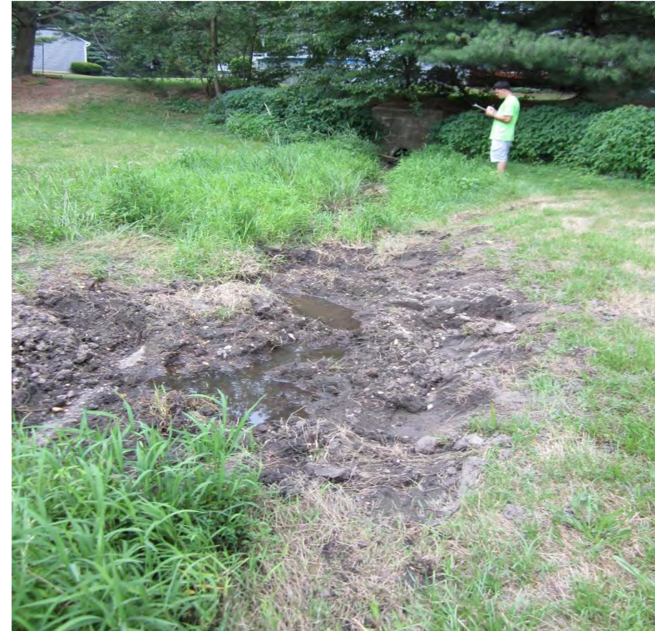
Clogged low flow and outlet.
