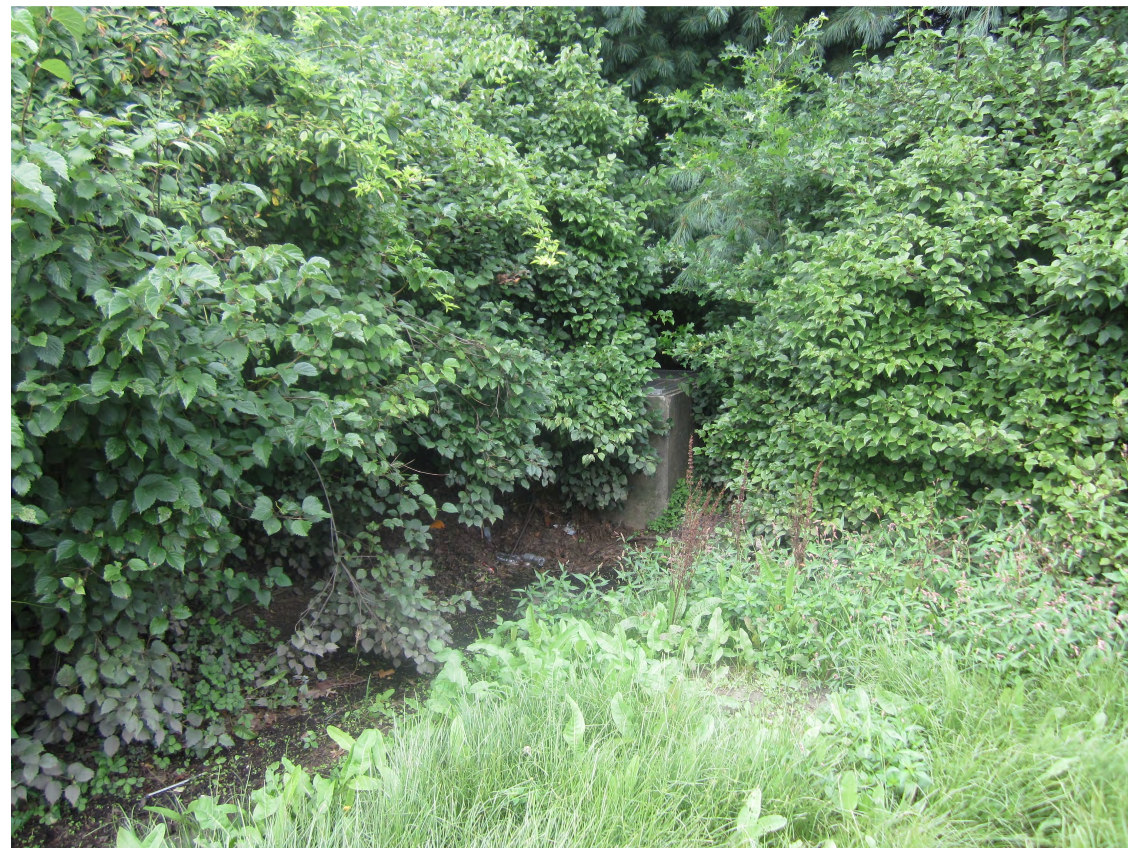
Overgrown outlet structure
