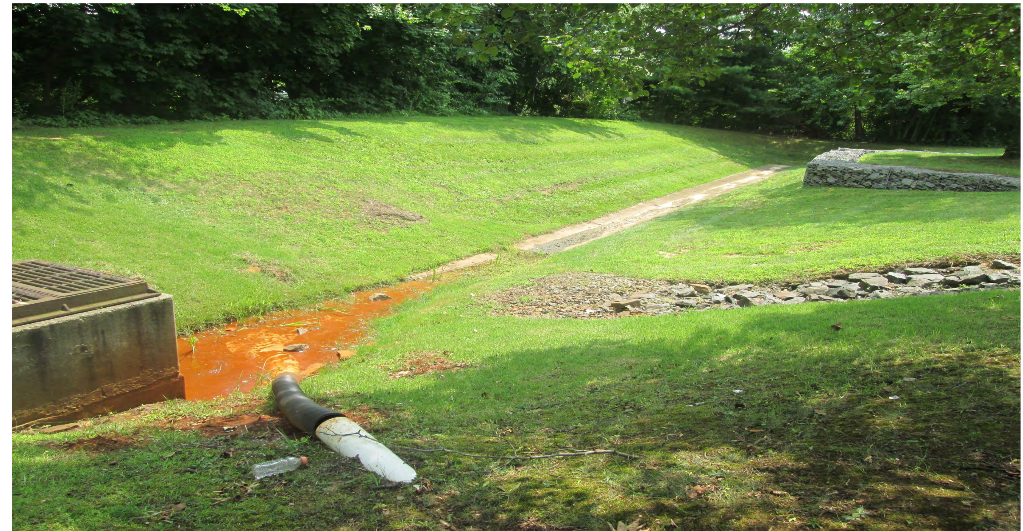
Overview of basin
