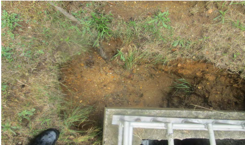
Erosion near outlet structure
