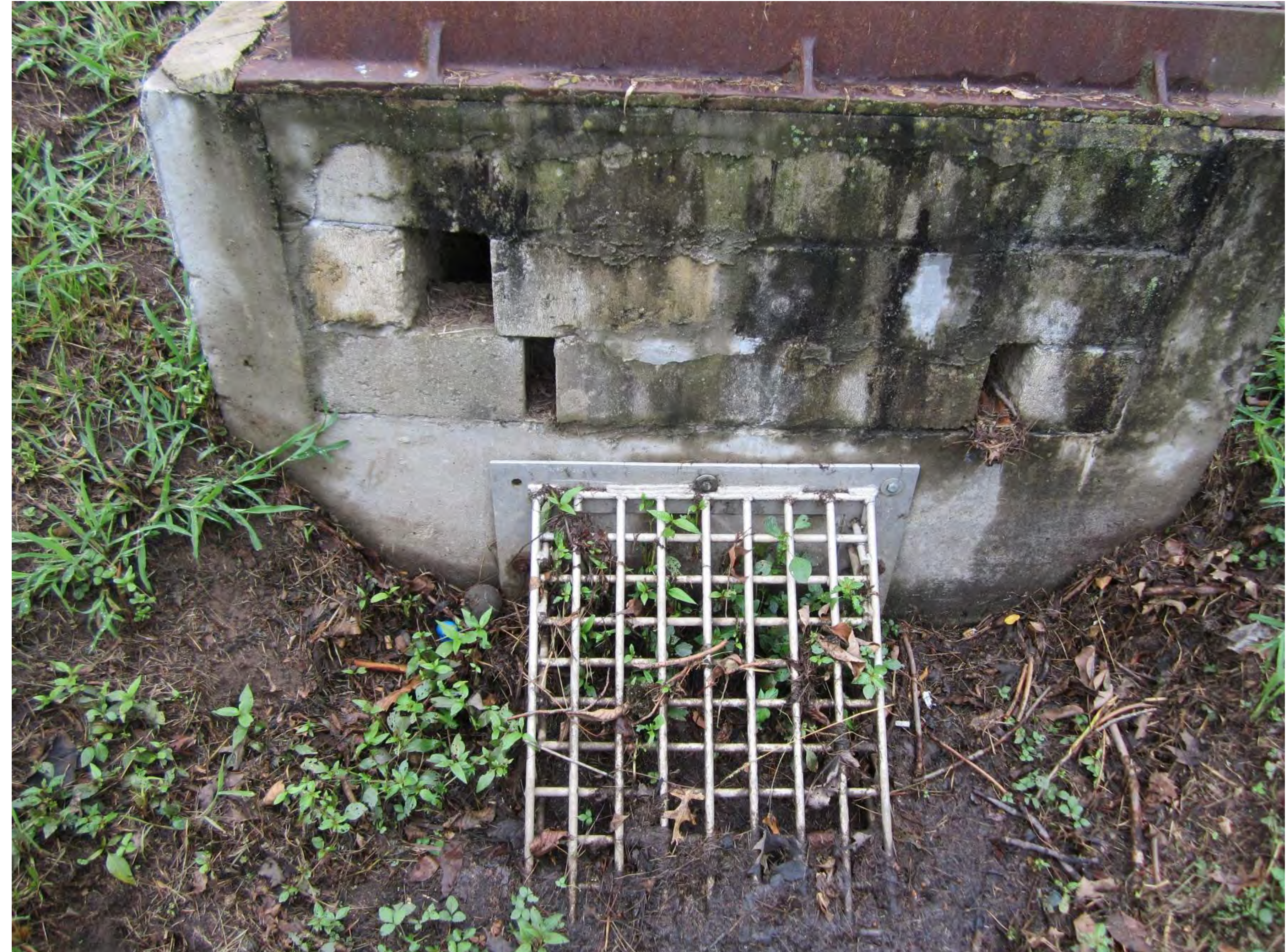
Clogged trash rack at outlet
