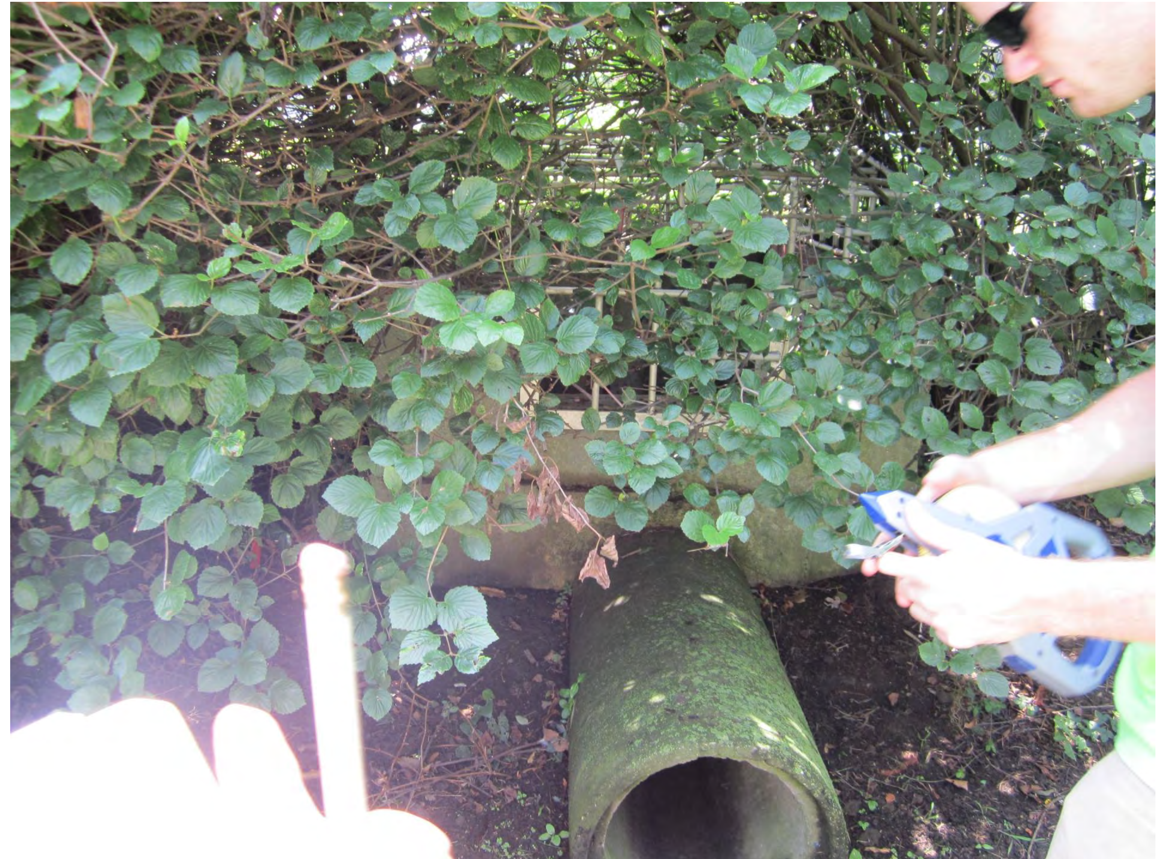
Woody vegetation growth around outlet
