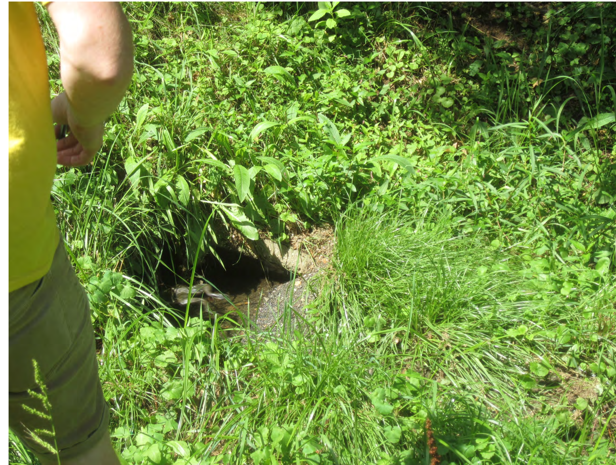
Southern inlet structure filled with sediment
