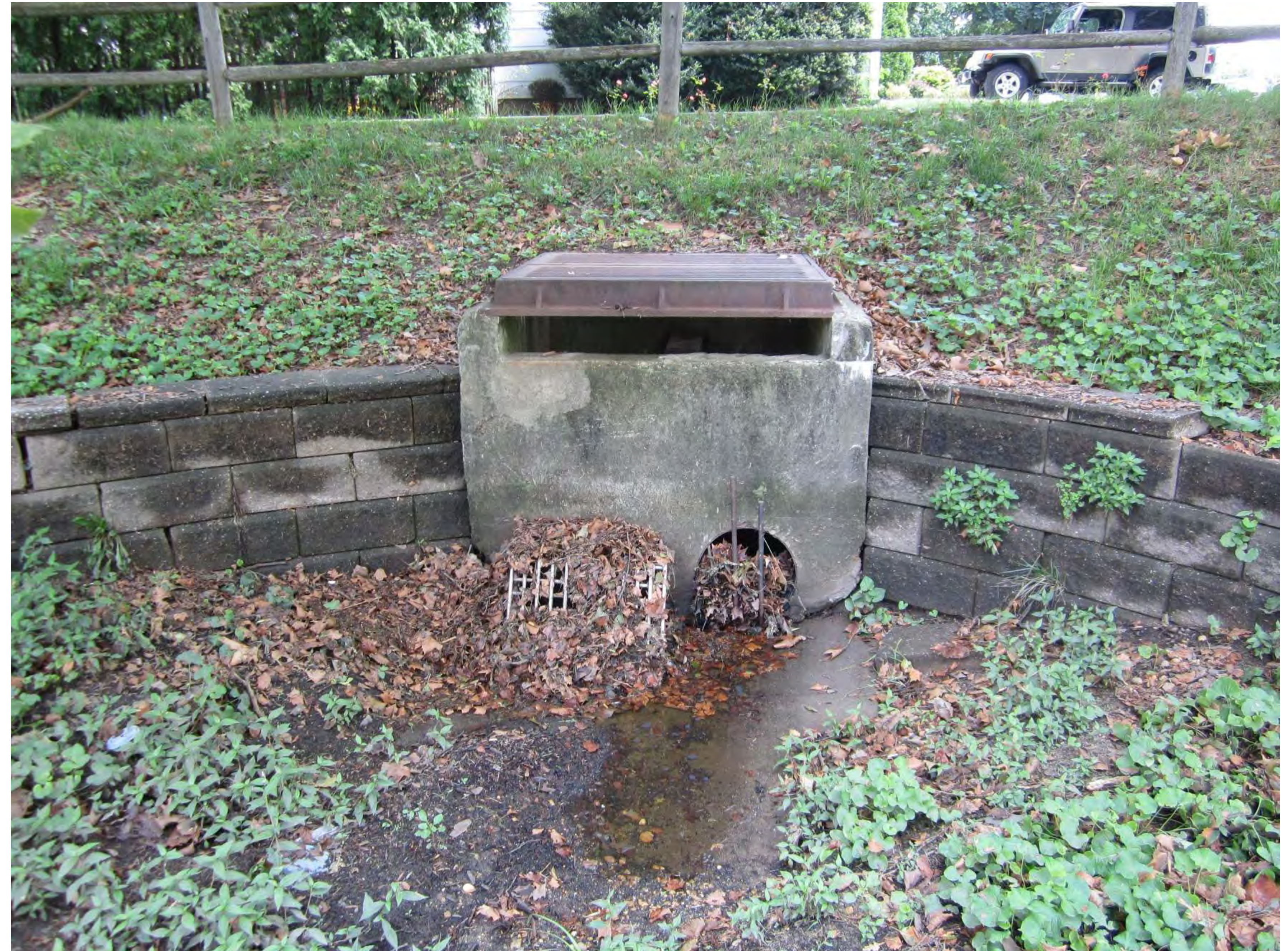
Clogged outlet structure
