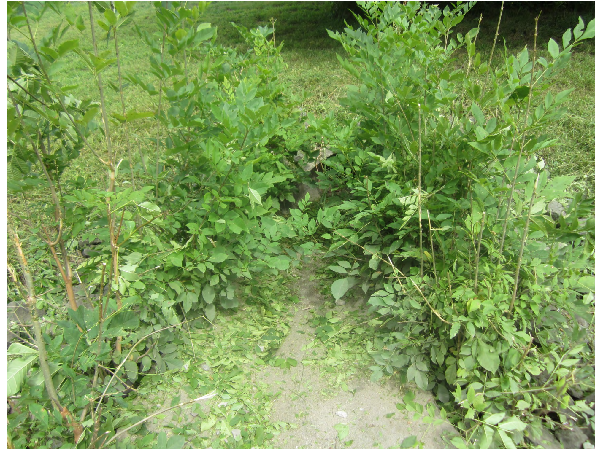
Overgrown inlet structure
