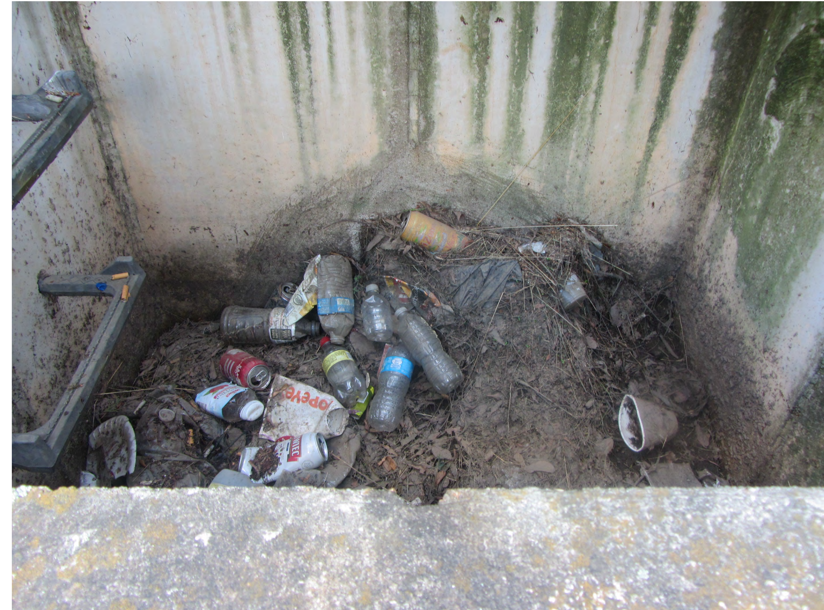
Litter and debris accumulated inside outlet
