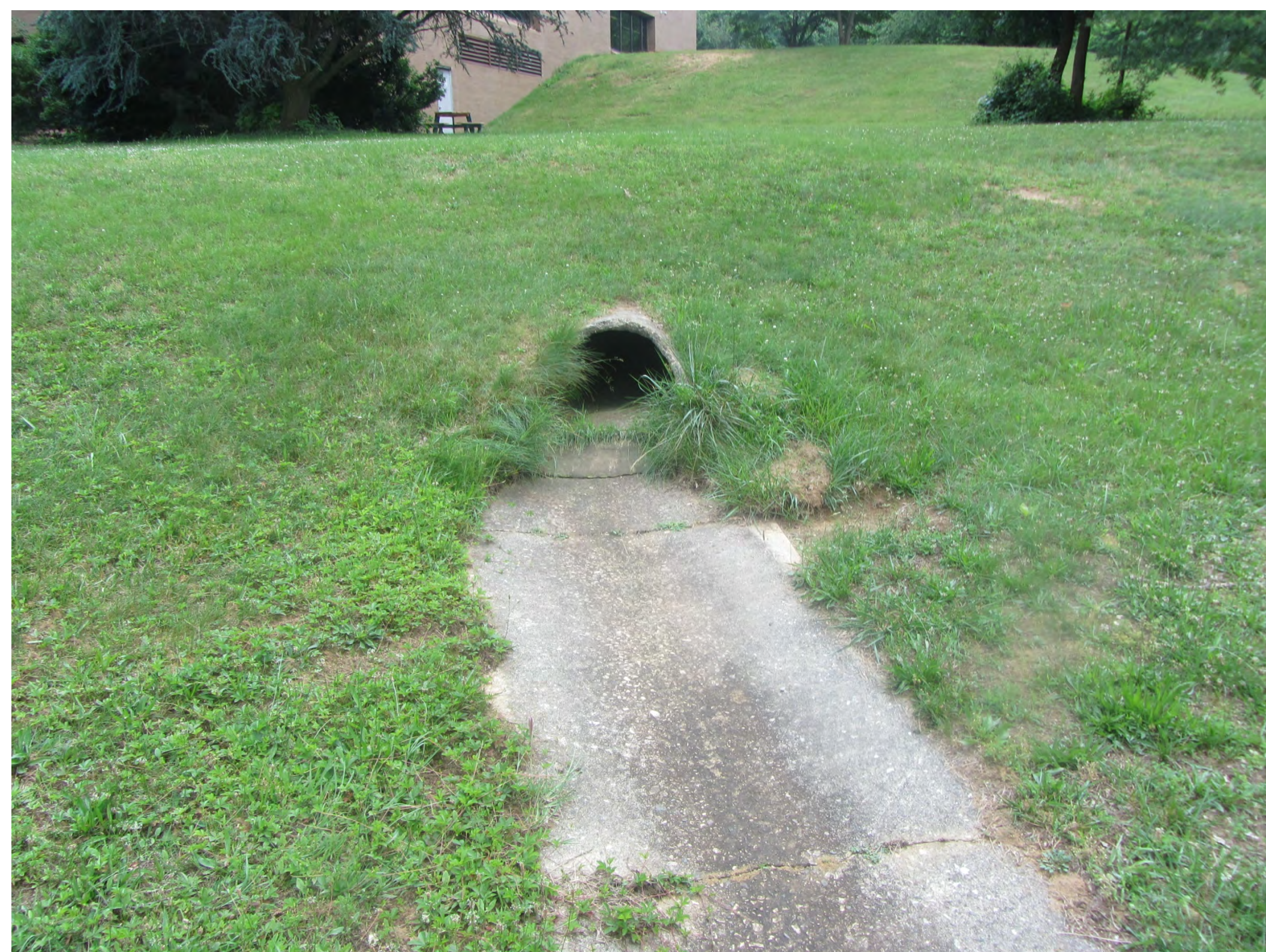
Concrete deterioration on northern inlet
