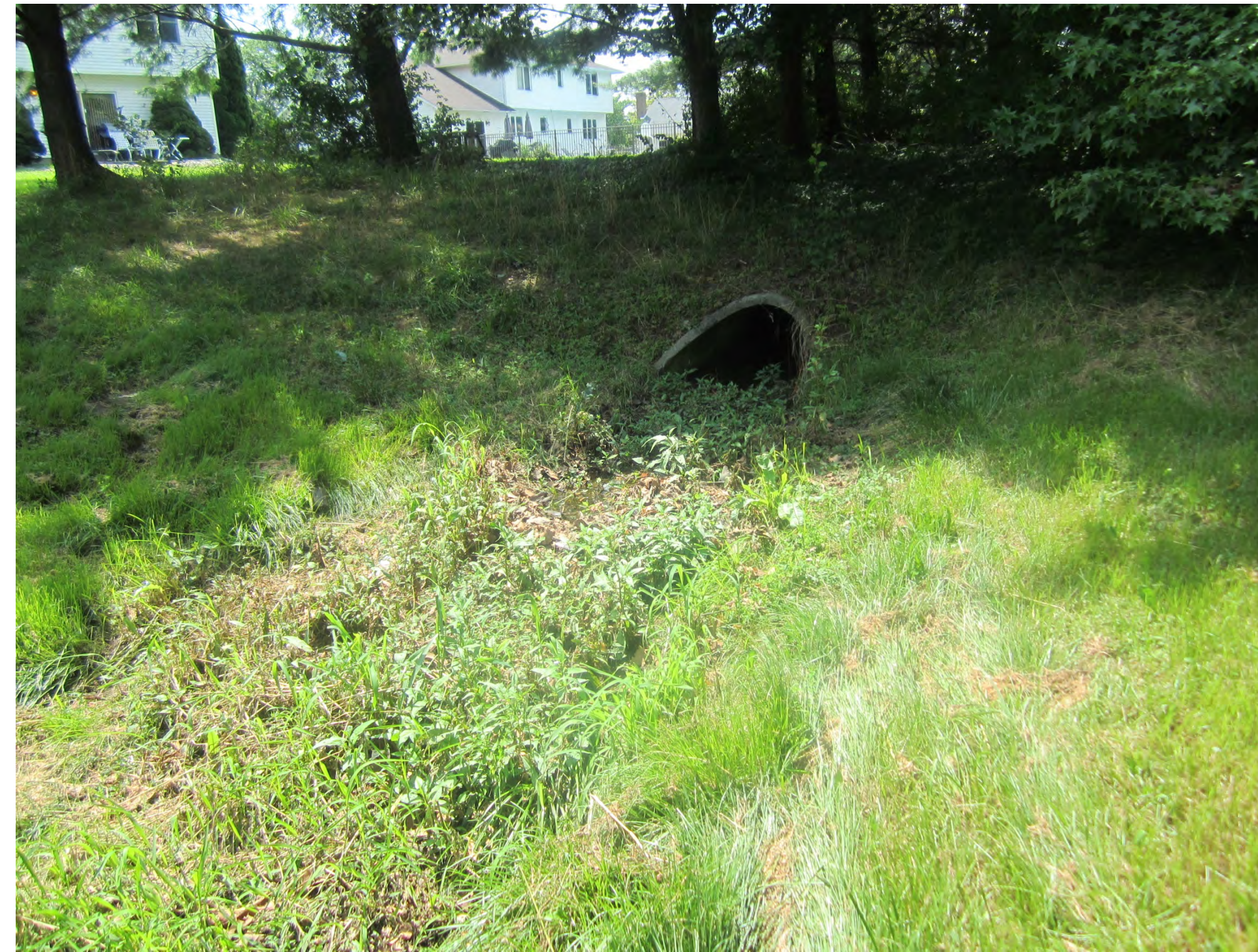
Excessive sediment in front of inlet
