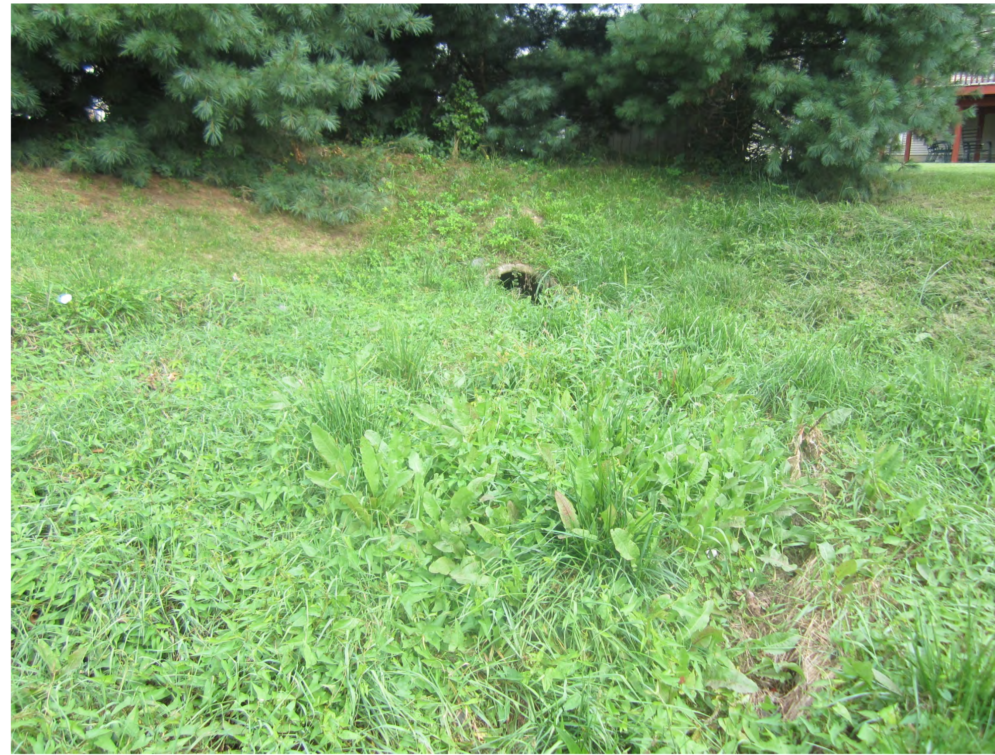
Inlet structure and overgrown rip-rap apron
