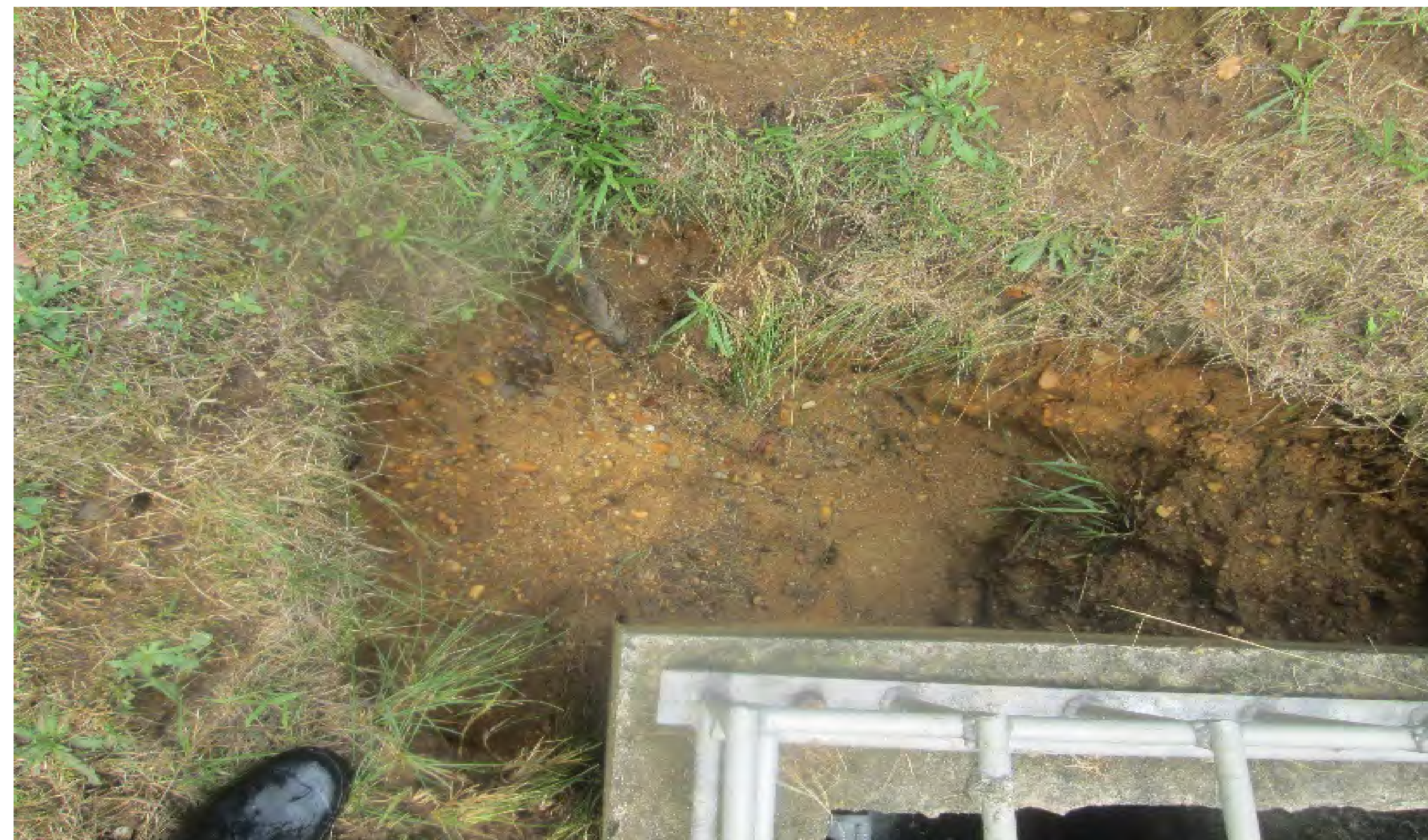
Erosion near outlet structure
