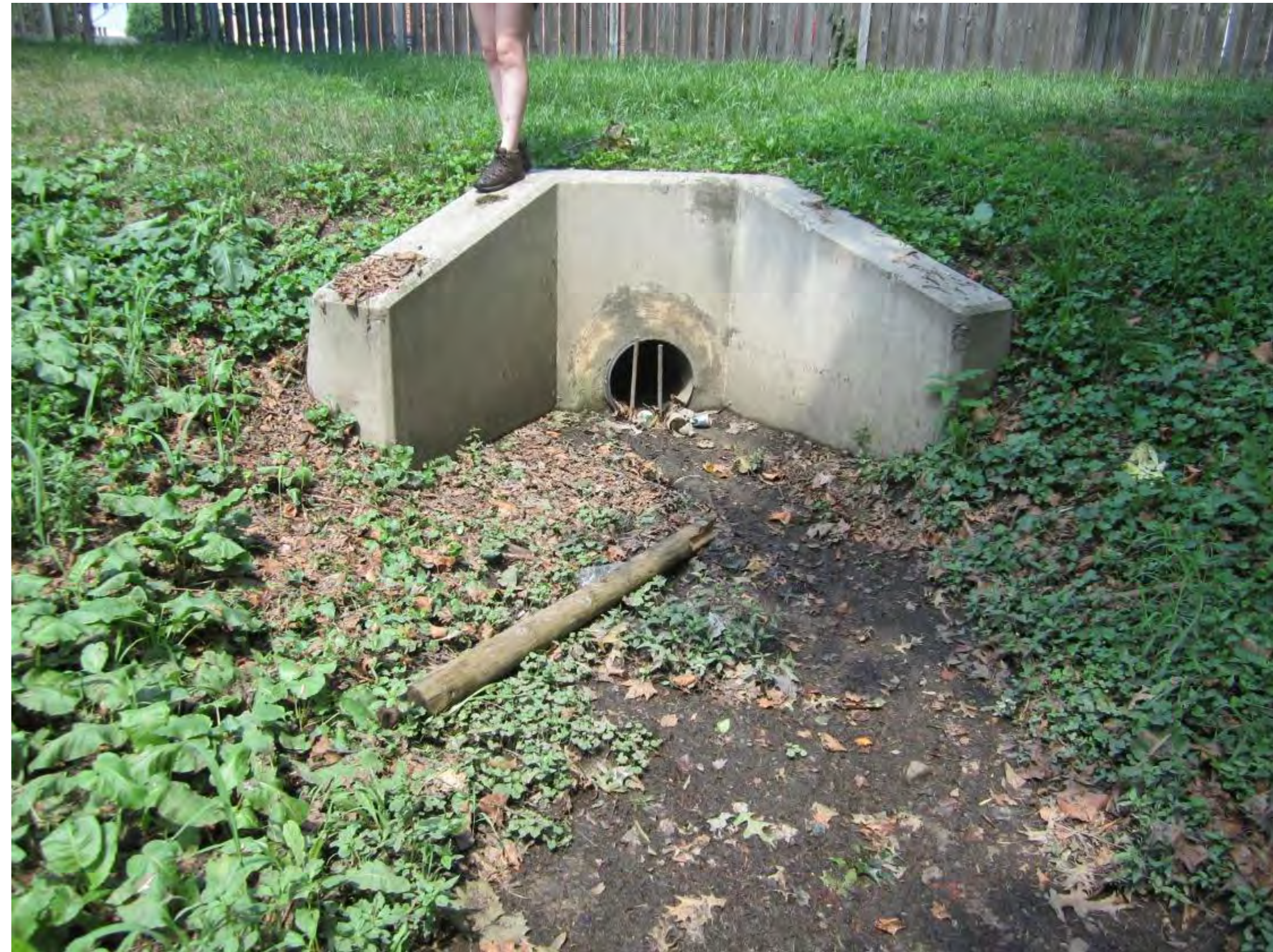
Inlet clogged with sediment
