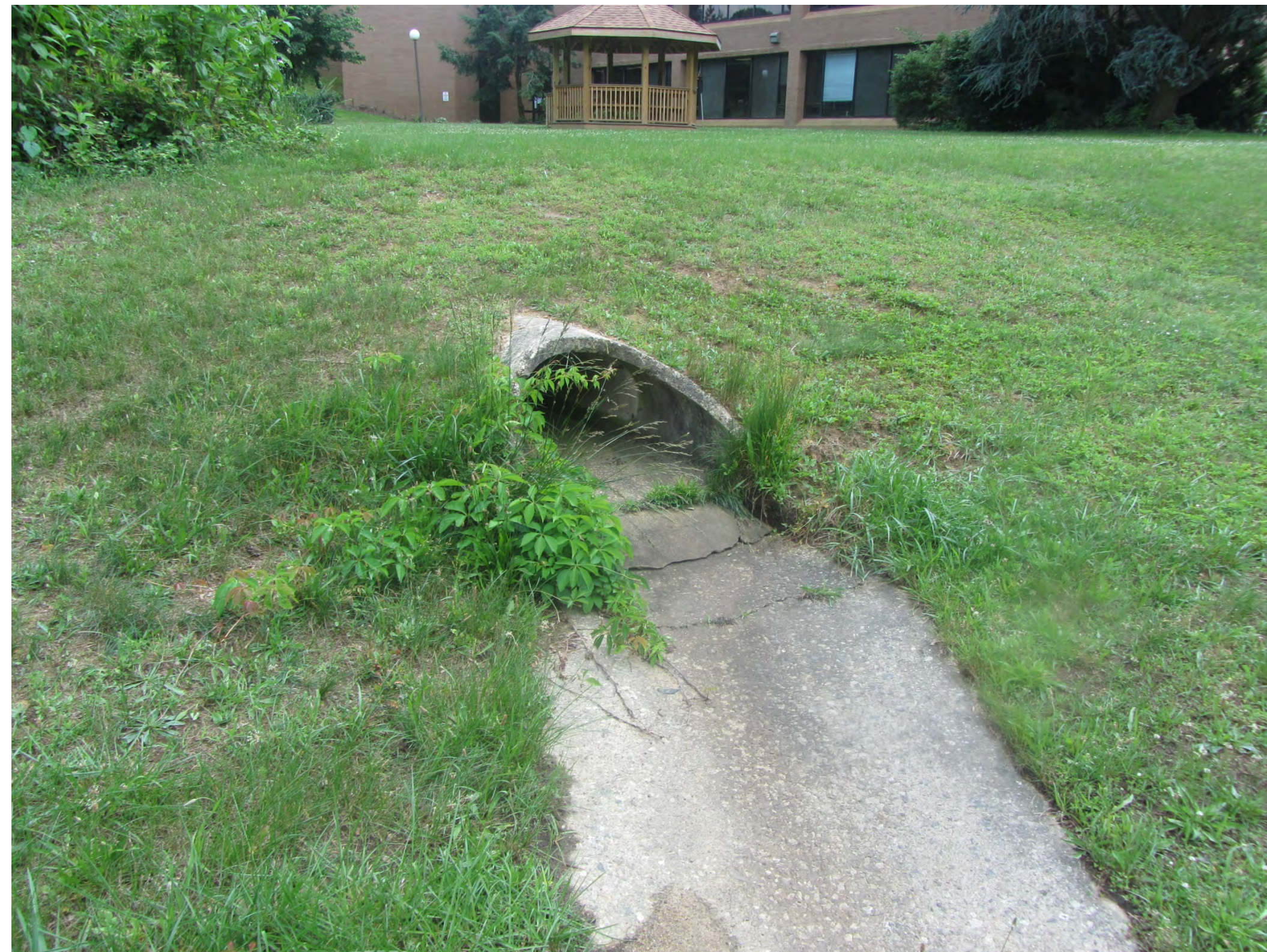
Concrete deterioration on southern inlet
