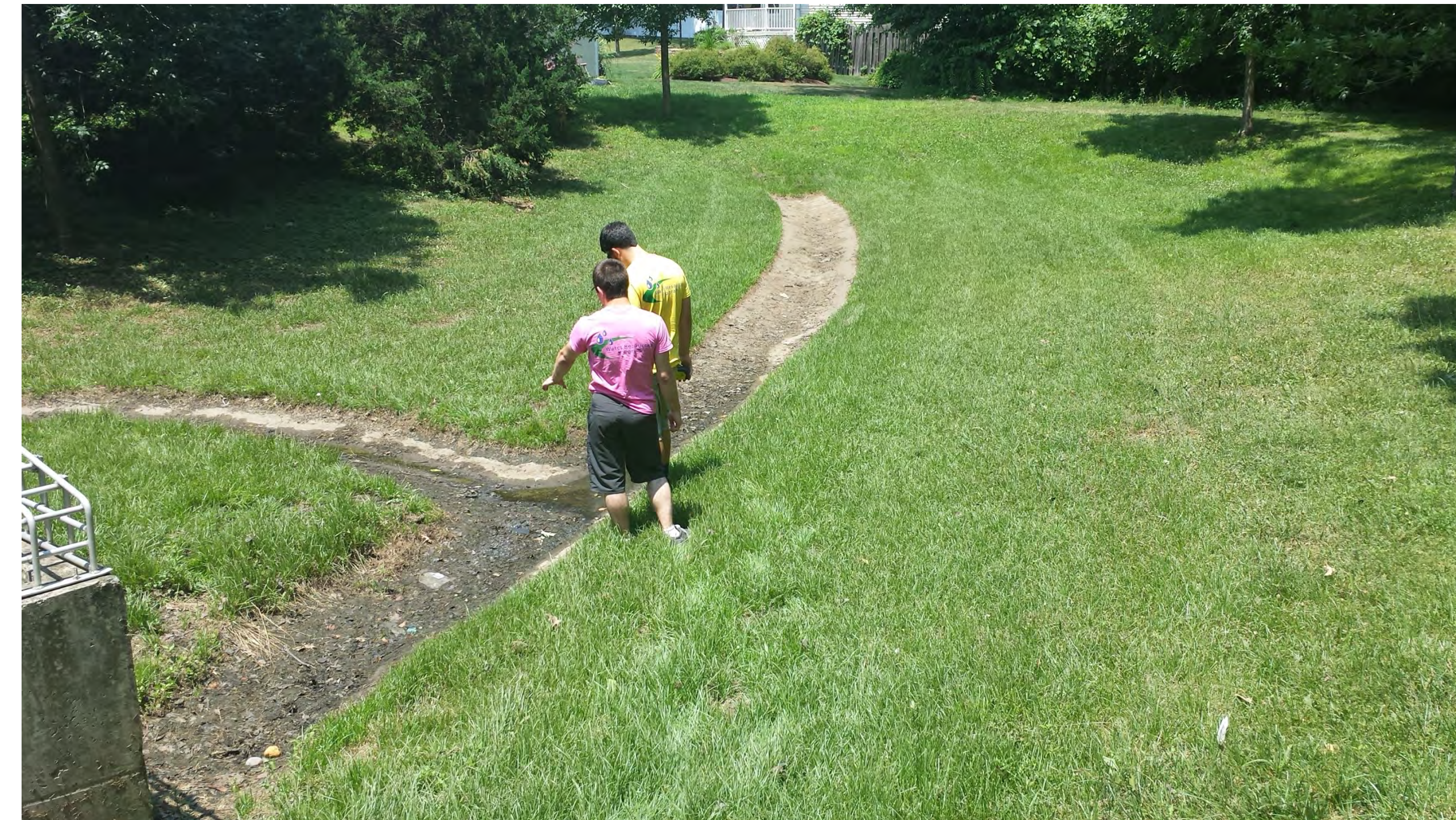
Sediment in low flow channel
