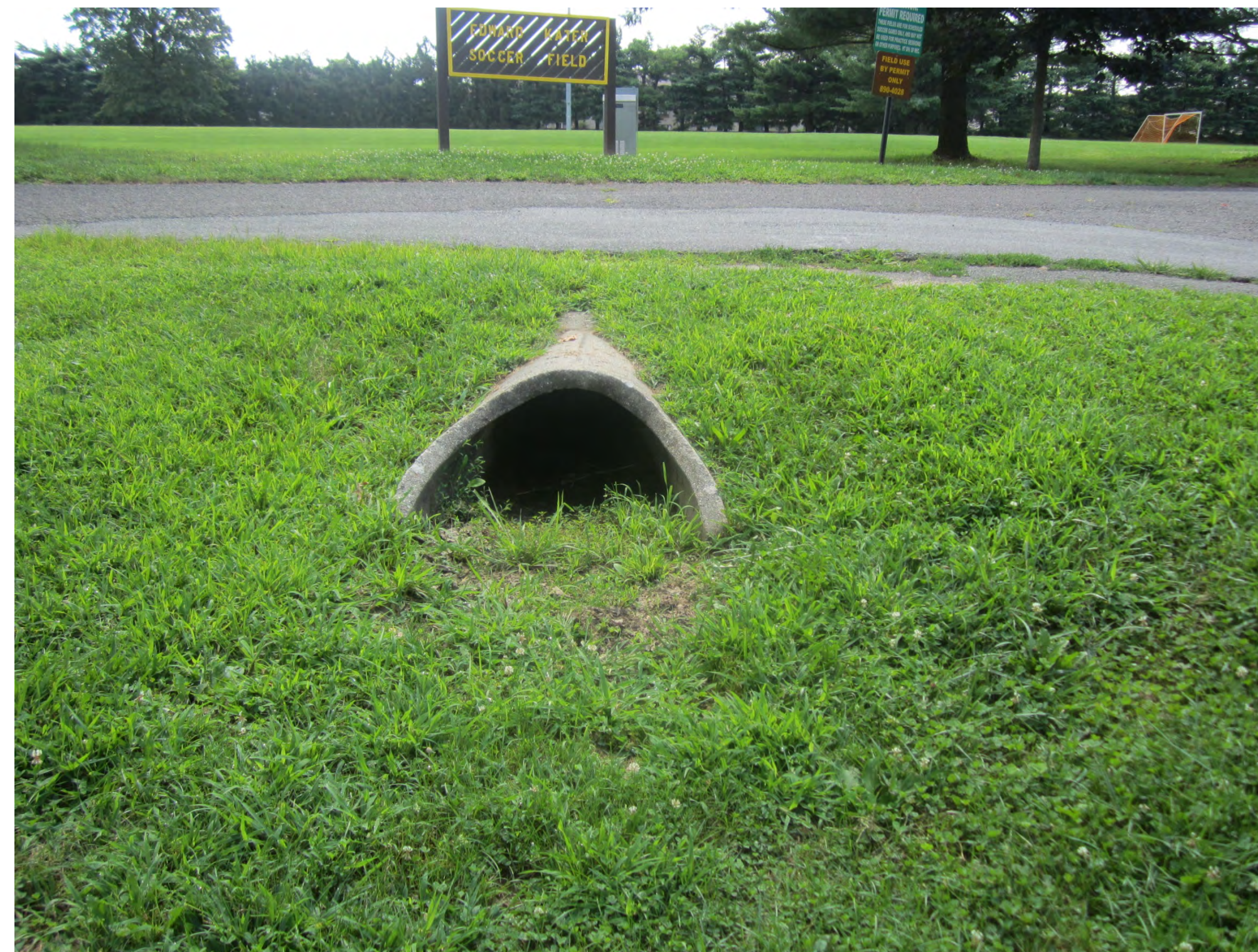
Basin #159 inlet structure
