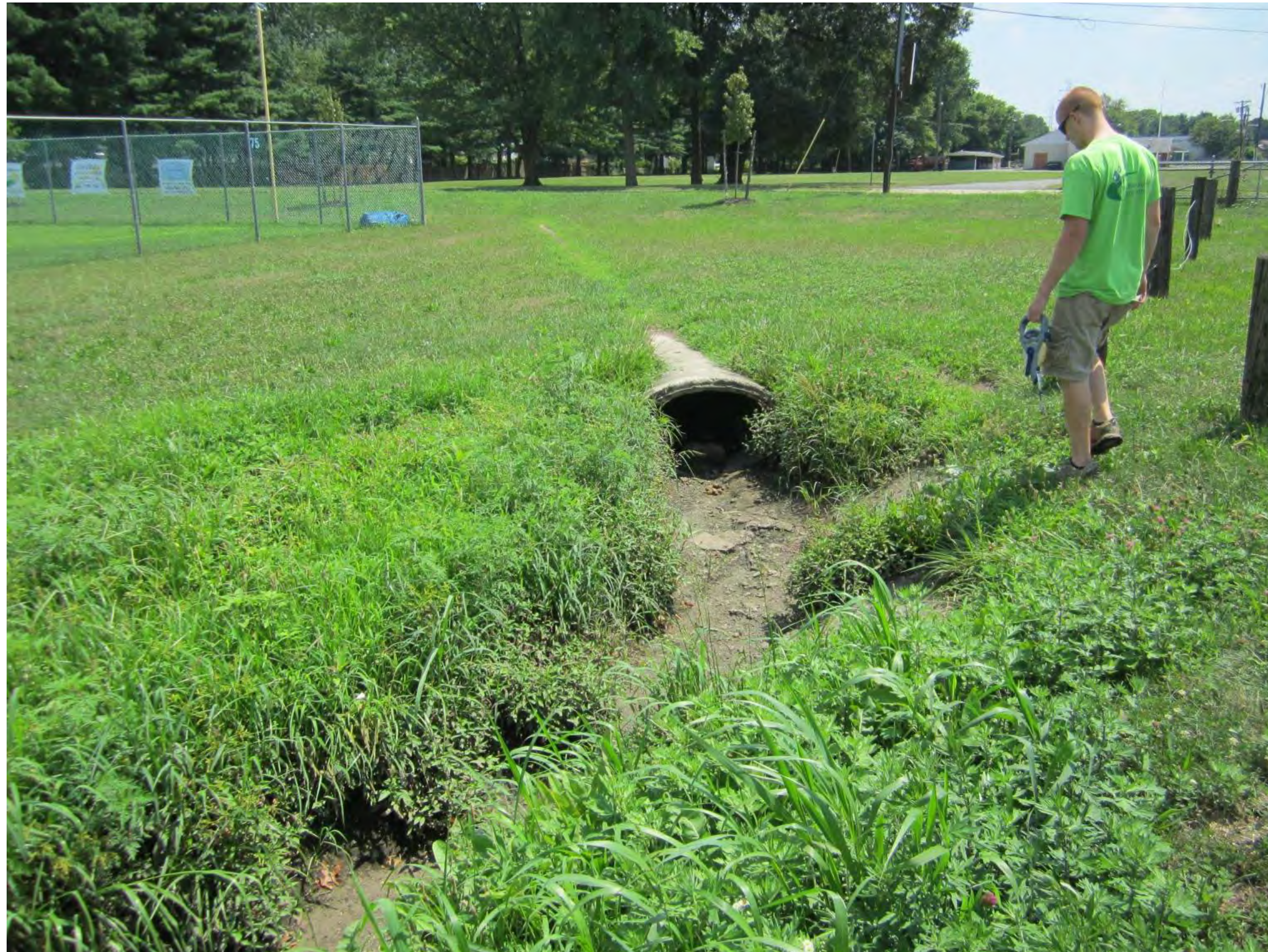
Inlet with sediment accumulation
