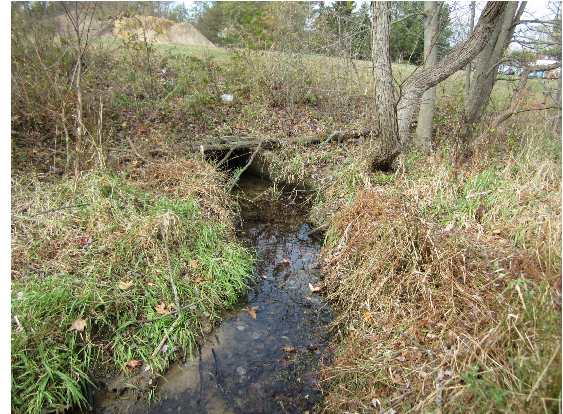
Inlet and erosion
