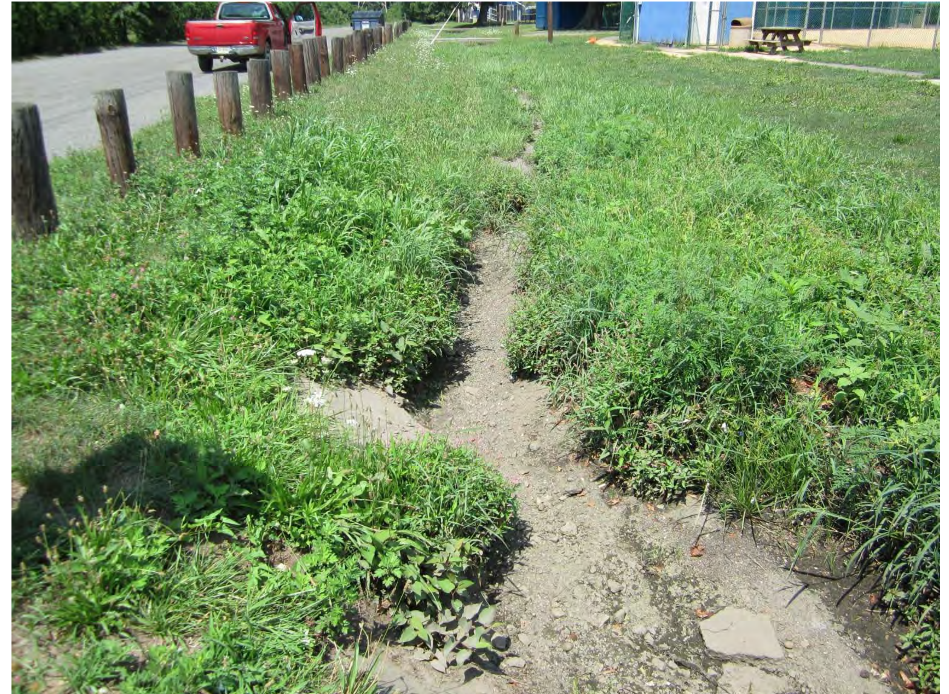
Basin bottom with erosion
