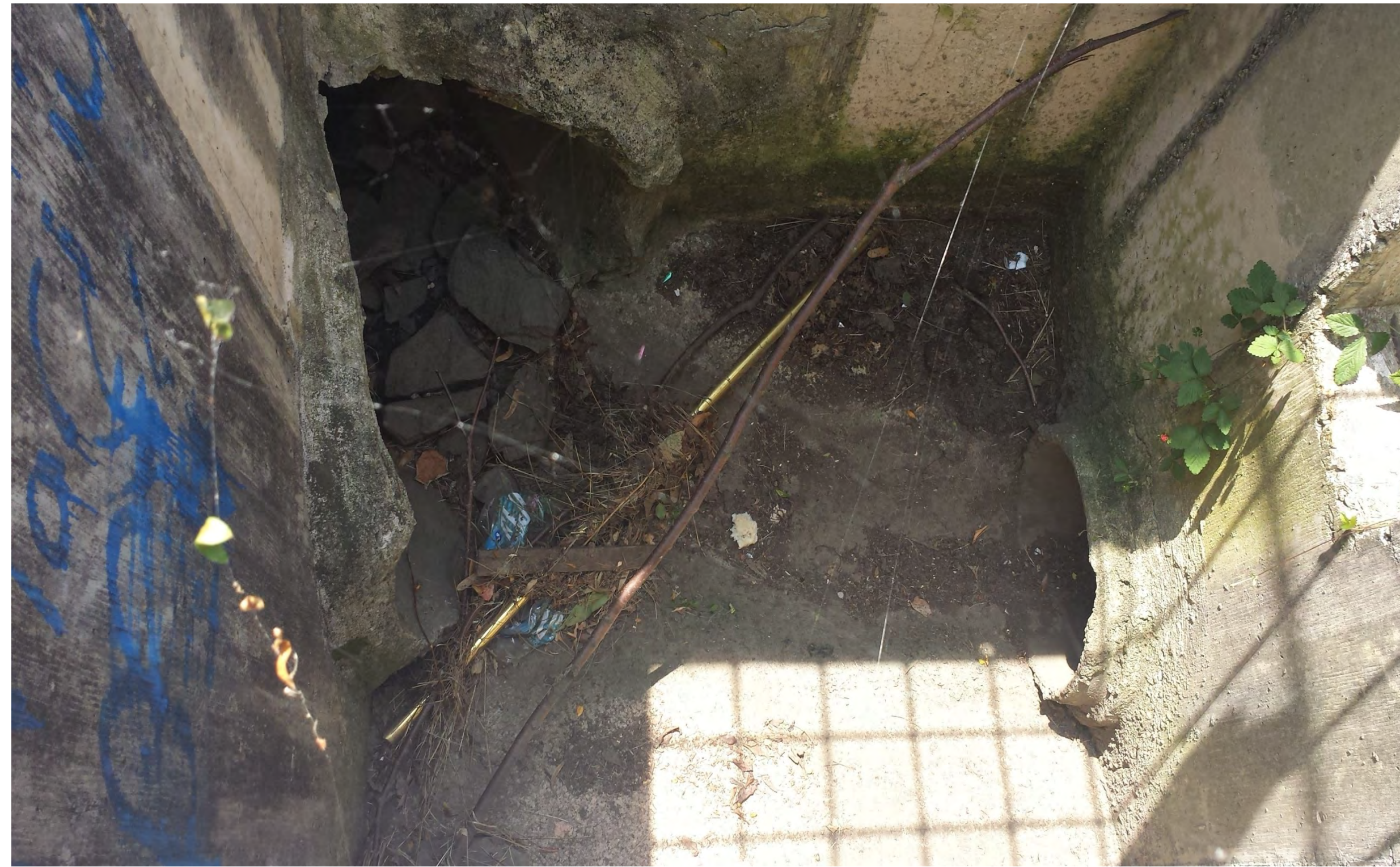
Inside of outlet
