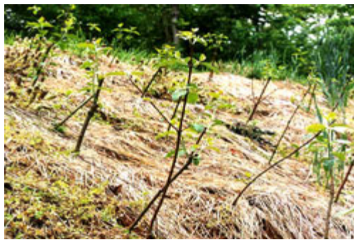
Figure 24: Erosion control and streambank stabilization with live stake plant material, North Carolina 3
