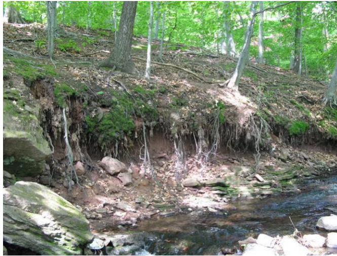
Figure 23: Example of an Eroded and Unstable Streambank in Musquapsink Brook Watershed
