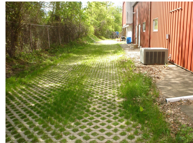
Pervious pavers at Parsippany-Troy Hills Department of Public Works facility Emergency Access Road. Note the downspout from the roof leading to the pavers. Photo credit Pat Rector, 5/2011
