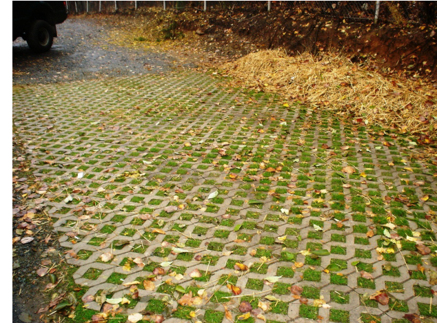
Grass Pavers at Parsippany-Troy Hills Department of Public Works Facility Emergency Access Road during a rain storm — note there is no runoff from the grass paver areas. Photo credit Pat Rector
