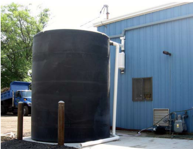
Figure 8b: A 5,000 gallon cistern used to disconnect the rooftop of the Department of Public Works in Clark Township to harvest rainwater for nonprofit car wash events
