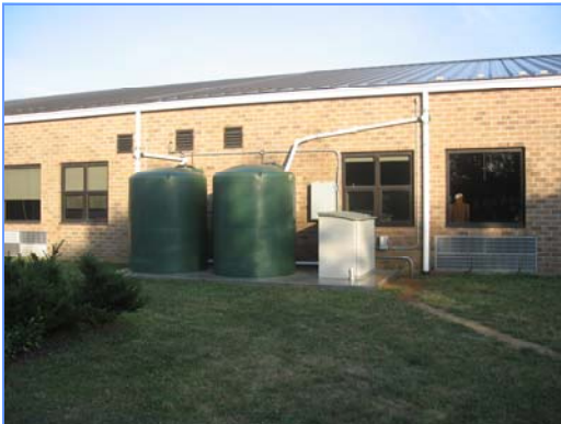
Samuel Mickle School Rainwater Harvesting System
