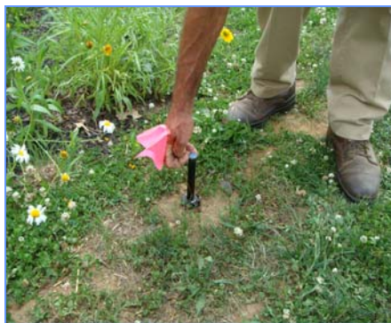
Newly installed sprinkler head at the Project WILD site at Samuel J. Mickle School.
