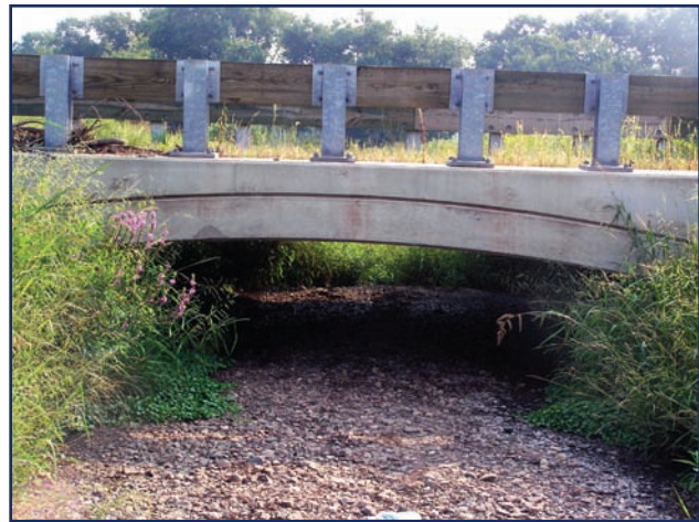
Figure 3~2. A culvert was replaced with this small bridge in Finderne Farms on the Raritan River.
