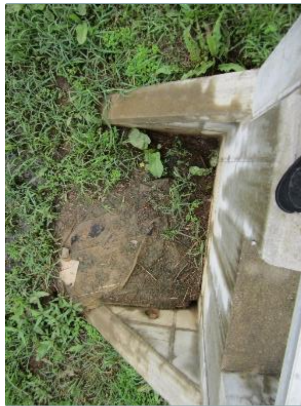
Outlet blockage by sediment
