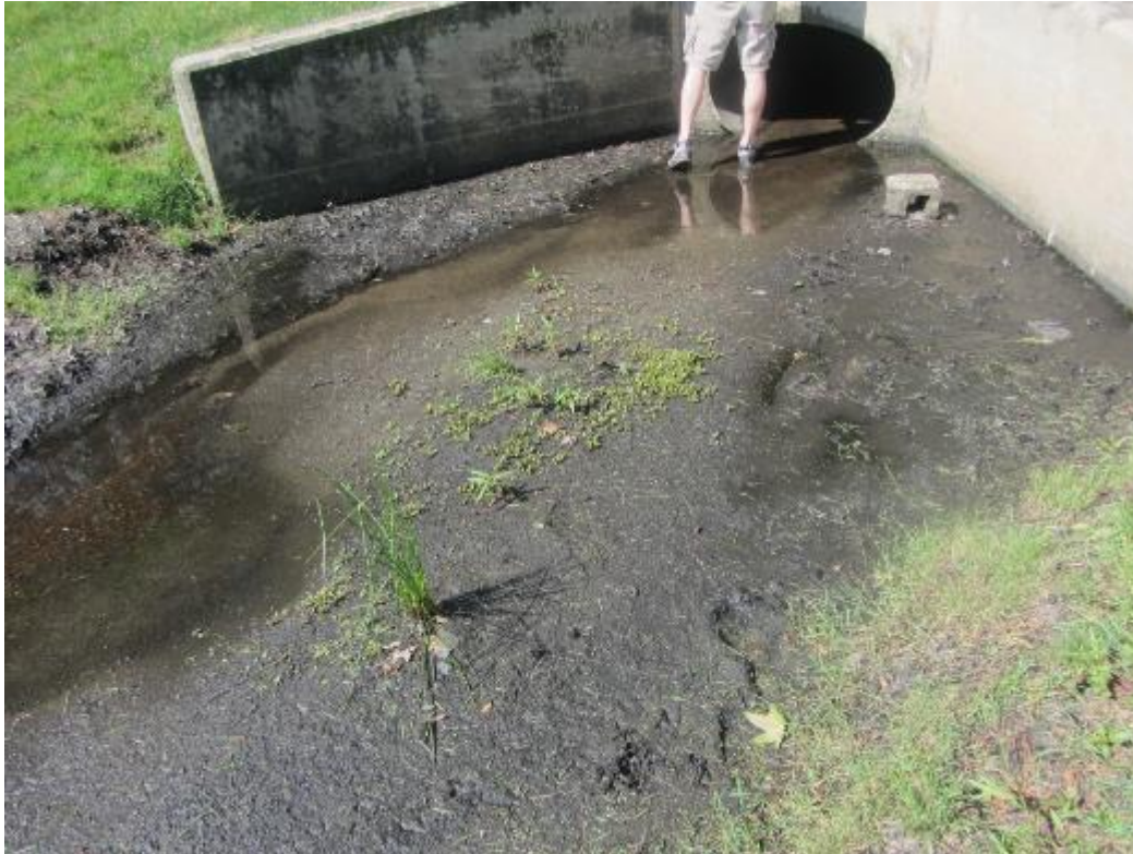
Accumulation of sediment in basin
