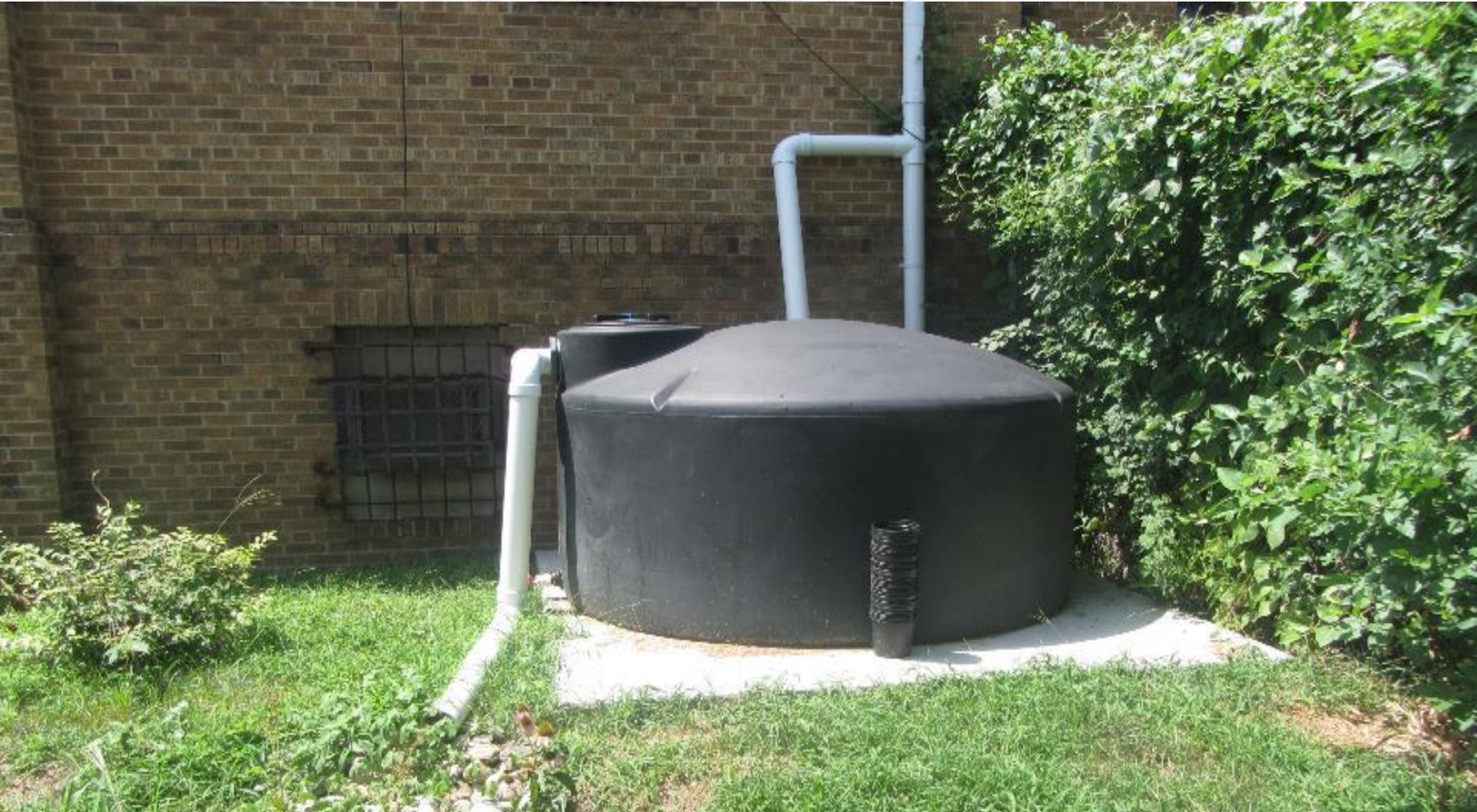
Cistern at the St. Bartholomew's Church Harvesting System
