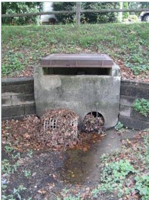
Outlet blockage by debris
