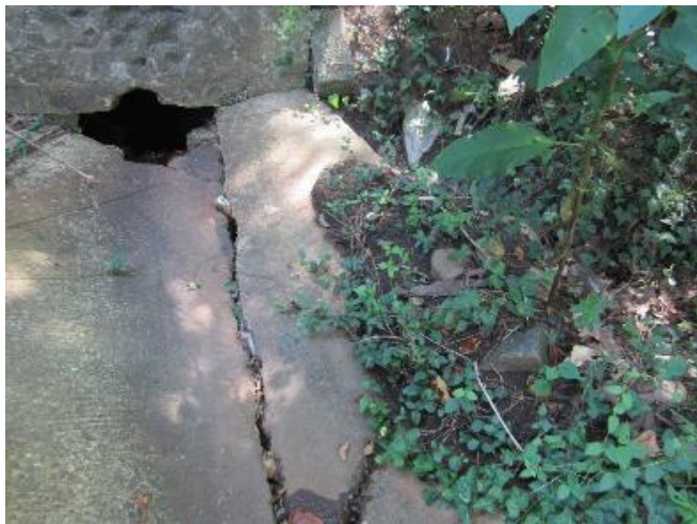
Broken low-flow channel
