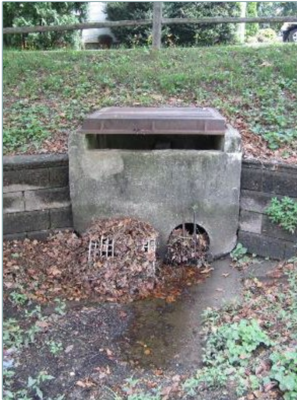
Outlet blockage by debris
