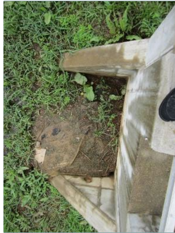
Outlet blockage by sediment
