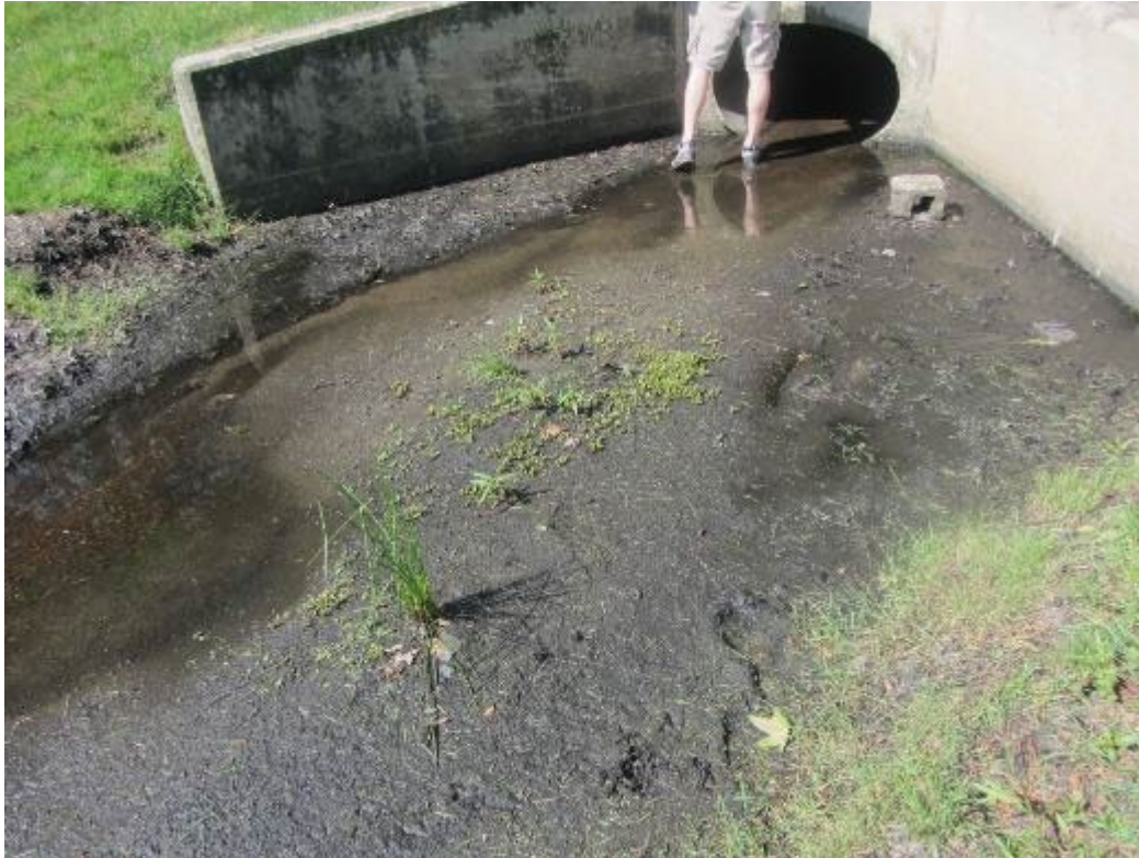
Accumulation of sediment in basin
