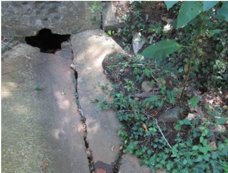
Broken low-flow channel
