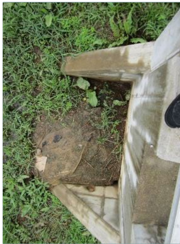
Outlet blockage by sediment
