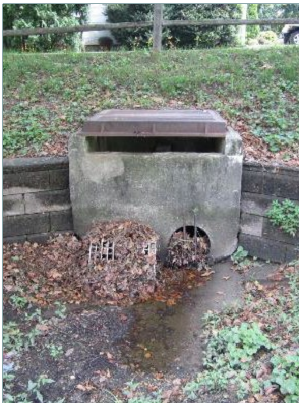
Outlet blockage by debris
