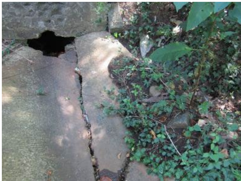
Broken low-flow channel
