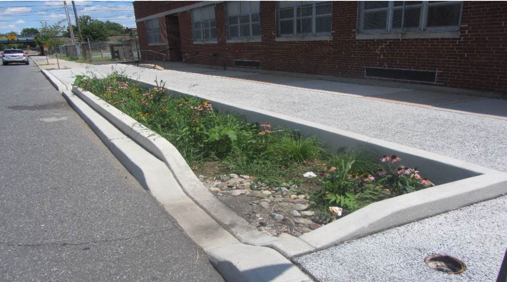
Stormwater Planter at the Brimm School
