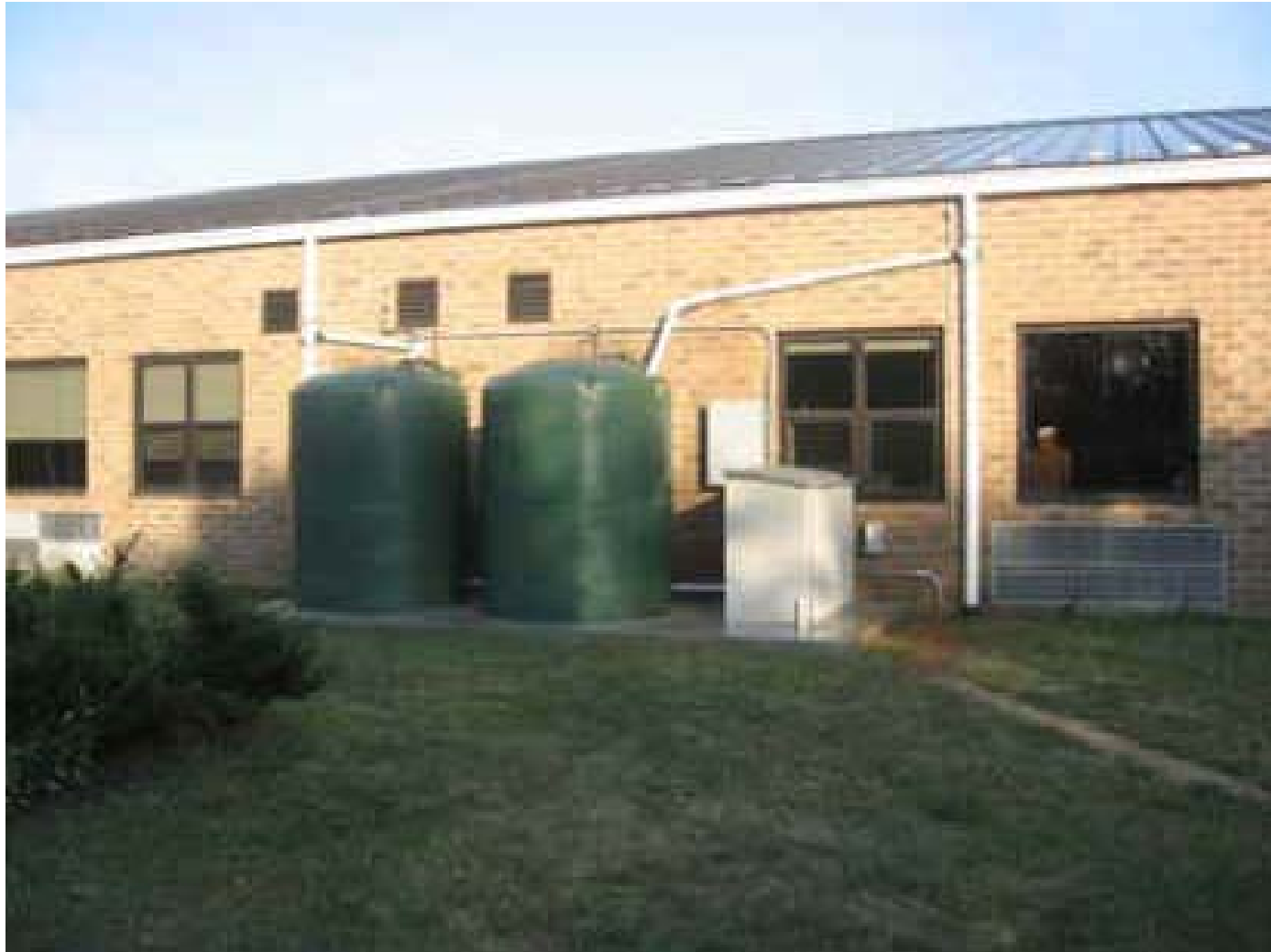
Samuel Mickle School Rainwater Harvesting System
