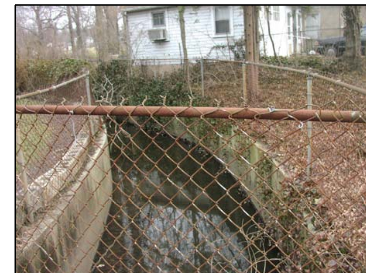
PICTURE 4: STREAM IS CONSTRICTED TO A 2 FOOT WIDE CONCRETE CHANNEL.
