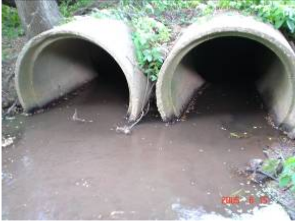
Figure 11a: Outfall pipes with turbid water along the Clarks Run. (Photo: RCE Water Resources Program)
