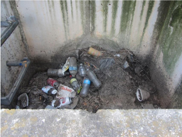
Accumulation of floatables from outfall
