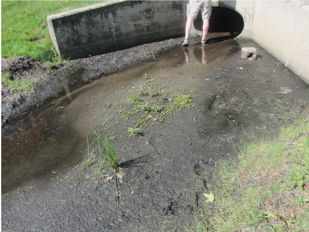
Accumulation of sediment in basin
