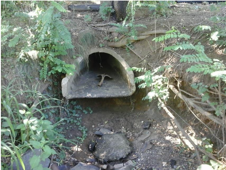
Outfall is causing erosion
