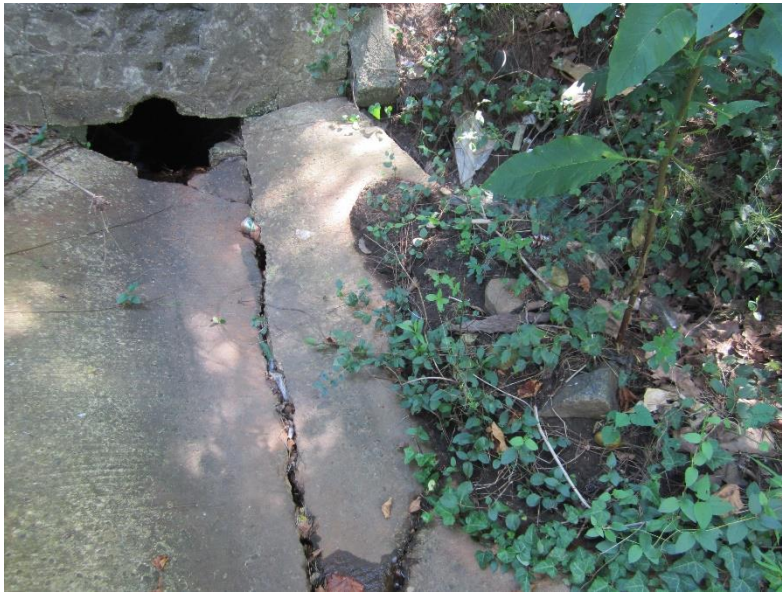
Broken low-flow channel
