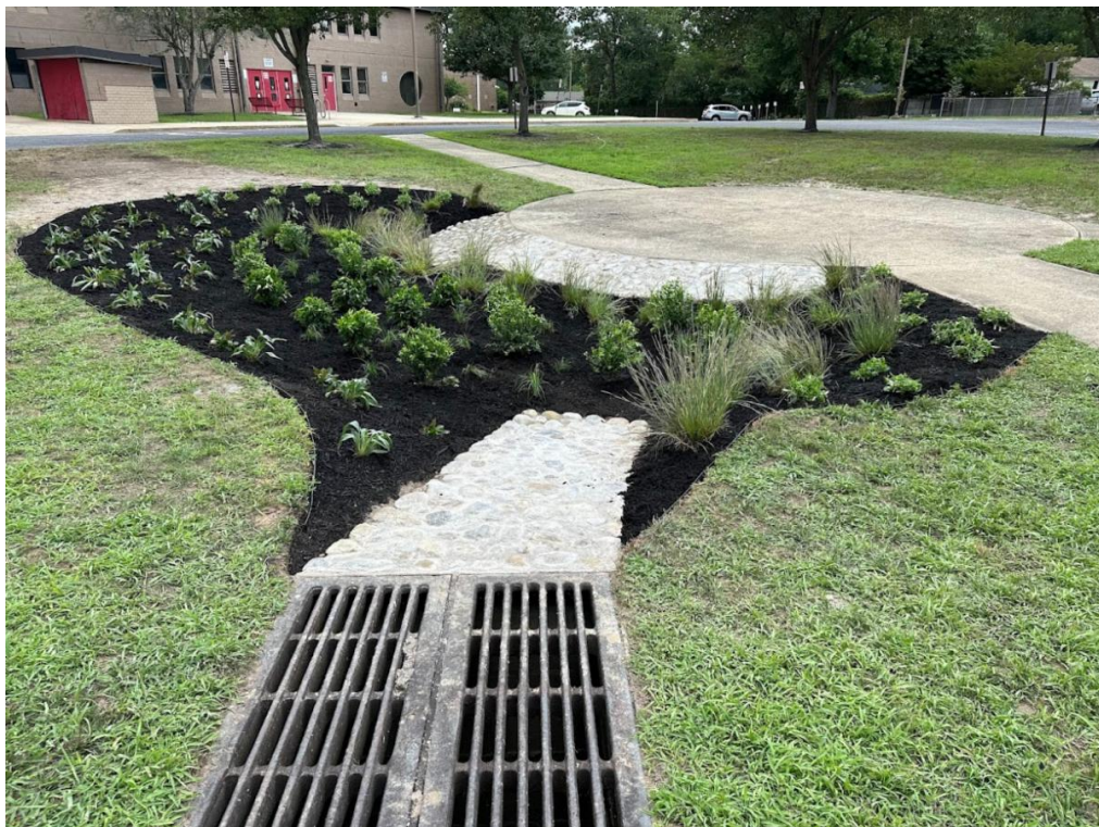
South Toms River Elementary School rain garden installation, July 24, 2024 [Photo credit: Hollie DiMuro, Water Resources Program]
