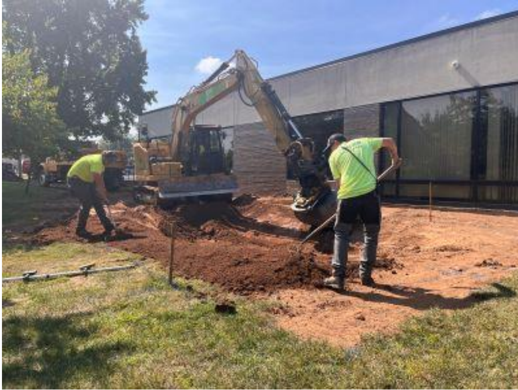
Construction of the Middlesex Public Library rain garden, September 2024 [Photo credit: Chris Perez, RCE Water Resources Program]
